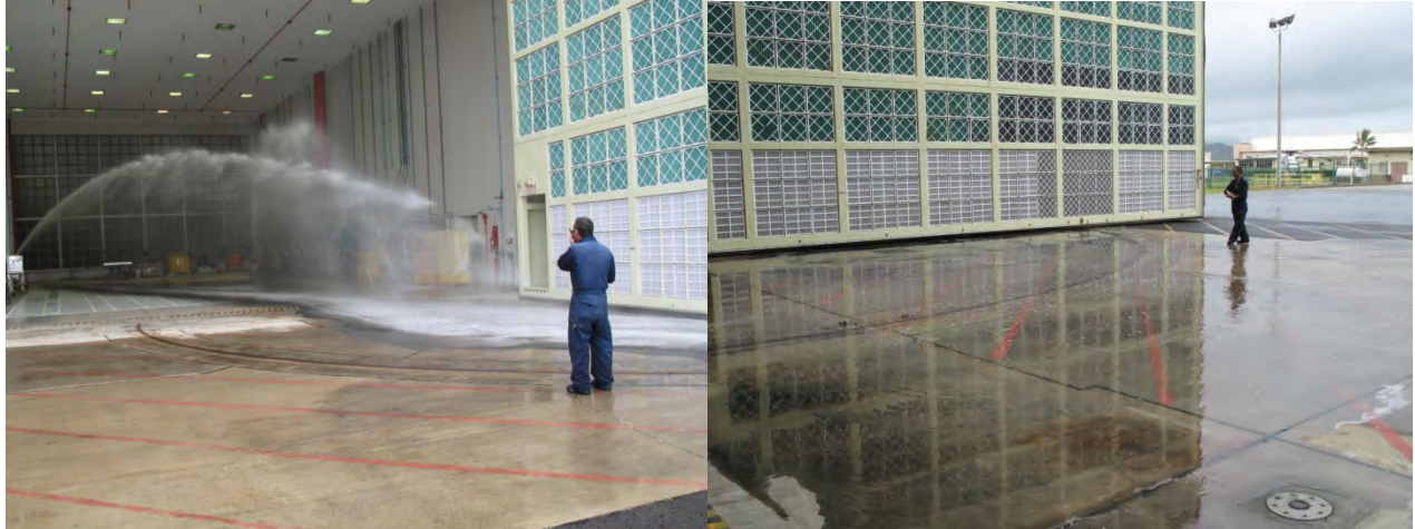
Figure 8. Result of MCB Hawaii NoFoam System Nozzle Discharge Check.
