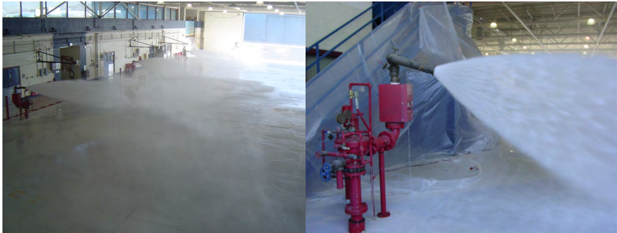
Figure 7. Result of Arizona ANG NoFoam System Nozzle Discharge Check.
