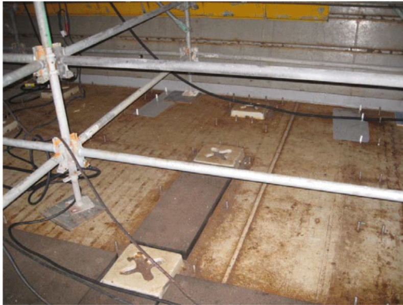
C. Deck Under Composite Material Beach Boards
