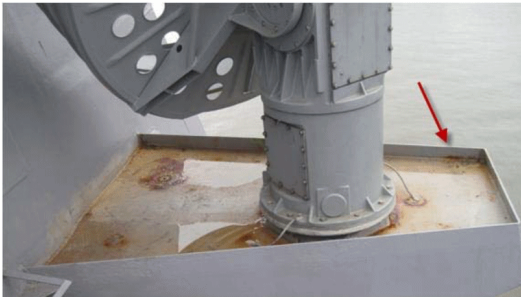
A. Coaming (Waterway Bar) Around Exterior Antenna Platform
