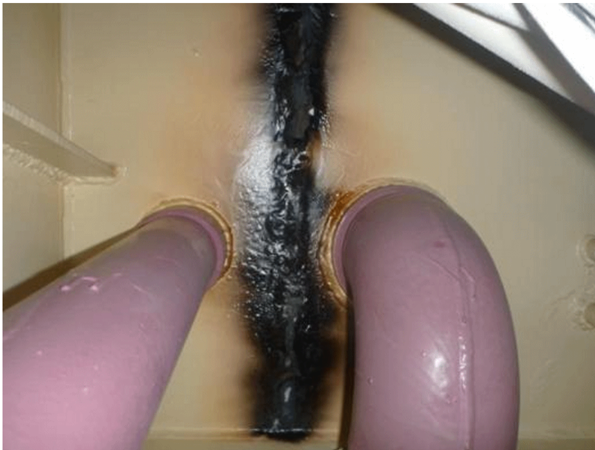
Figure 6-1 Burned Coating From Welding on Opposite Side of Plate
