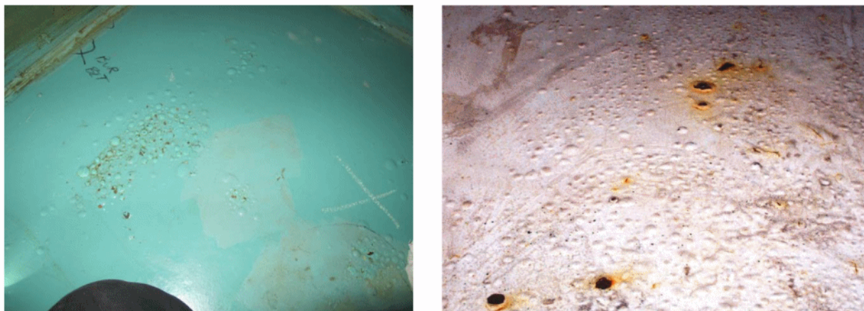
Figure 4-13 Examples of Osmotic Blistering Found in In-Service Tanks
