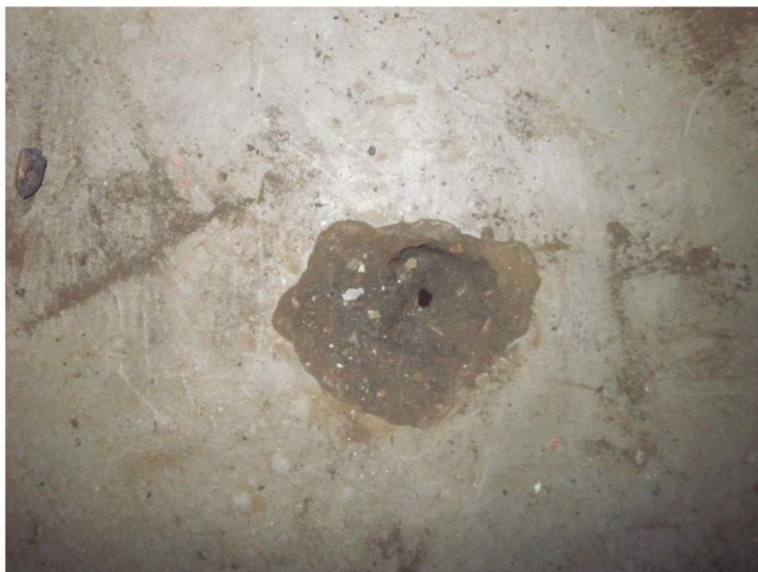
Figure 4-18 Examples of MIC-Produced Isolated Pitting in a Waste Oil Tank
