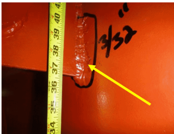
Undercut Base Metal At Weld Toe
