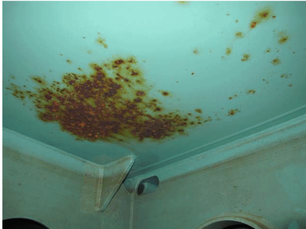
A. Corrosion in ballast tank overhead (tank top) above the waterline
