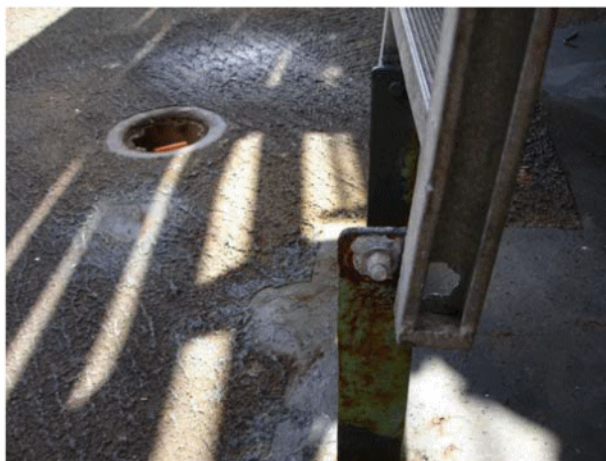
Aluminum Ladder and Steel Supports
