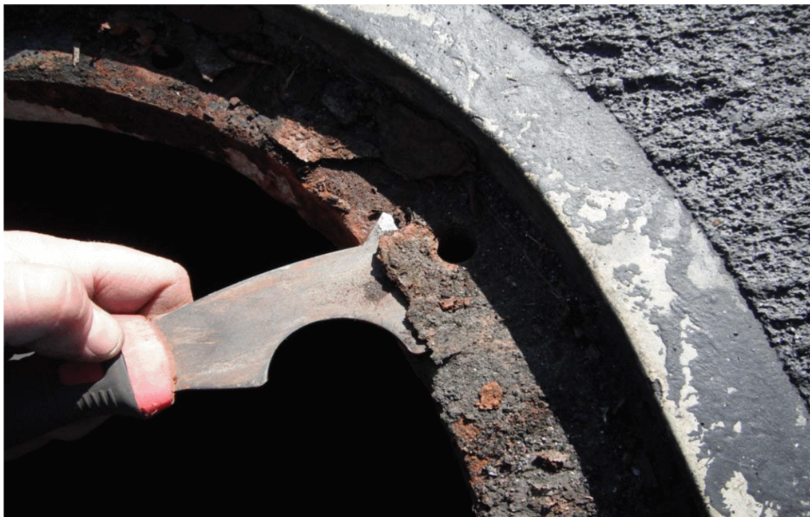
Figure 4-6 Heavy Rust Scale Of Steel Deck Manhole Cover Seating Surface
