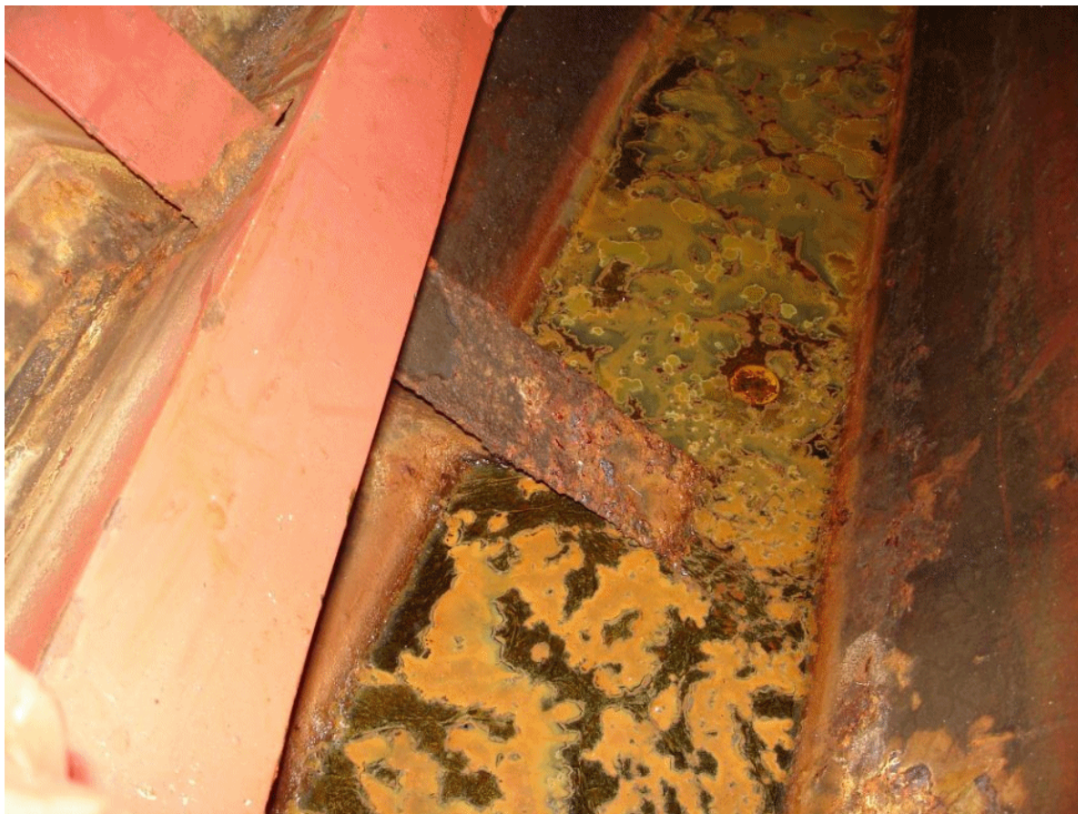
Figure 1-4 Bilge Pocket Obscured by Oily Water and Sludge
