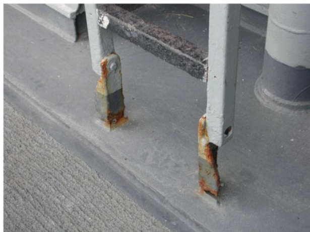
GRP Ladder and Steel Supports
