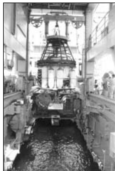
Figure 1-20. PTC Handling System, Elk River .
