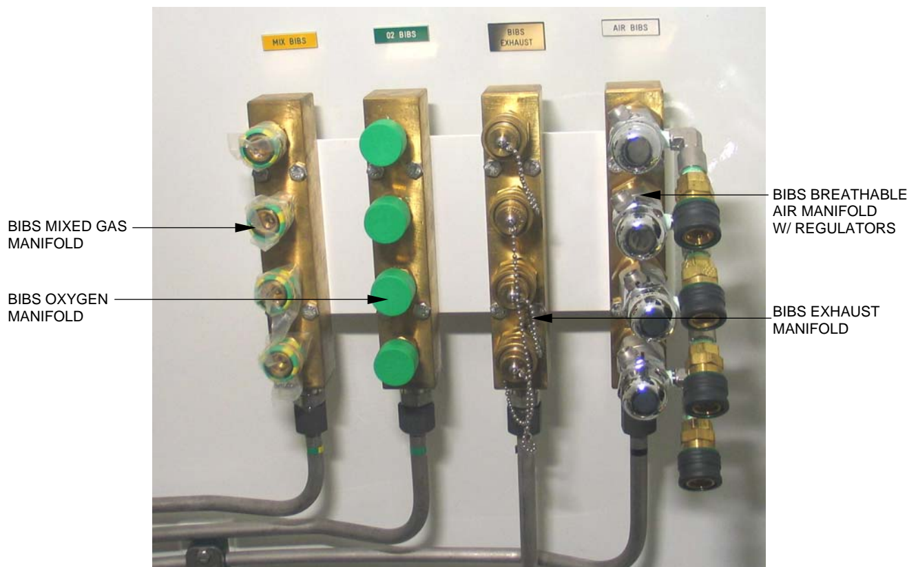
Figure 3-19. BIBS Manifolds (Inner Lock)
