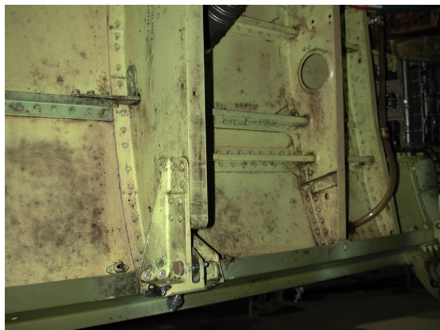
Figure 3-30. Biological Growth on Helicopter Wall
