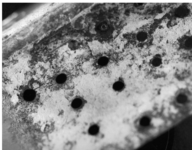
Figure 3-23. Aluminum Surface Corrosion Products
