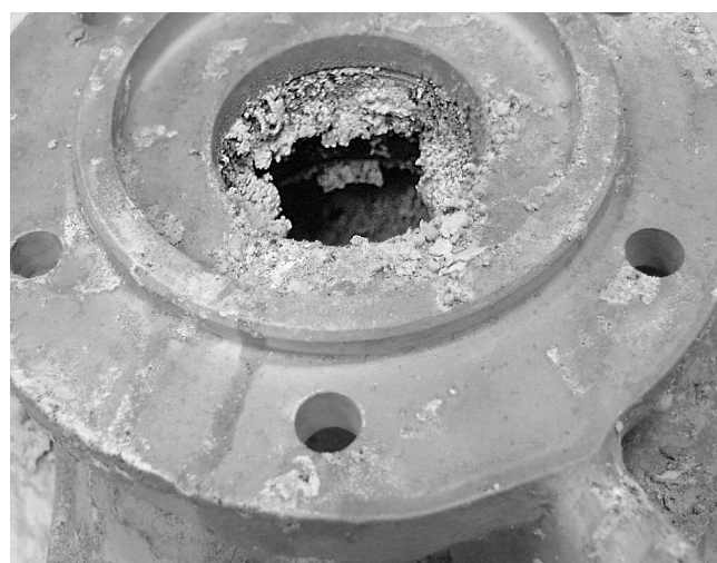
Figure 3-24. Magnesium Corrosion Products
