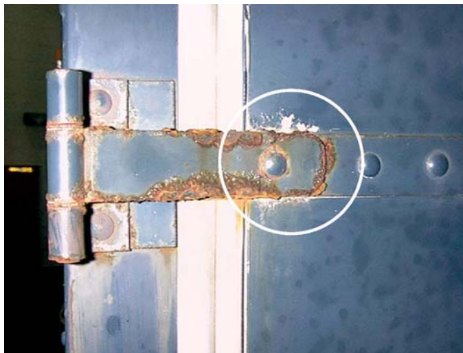
Figure 1-6. Example of Galvanic Corrosion - Steel Hinge Bolted to an Aluminum Door
