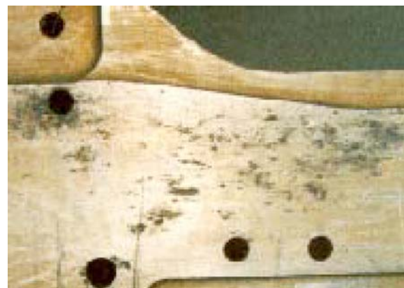
Figure 1-7. Example of Pitting Corrosion
