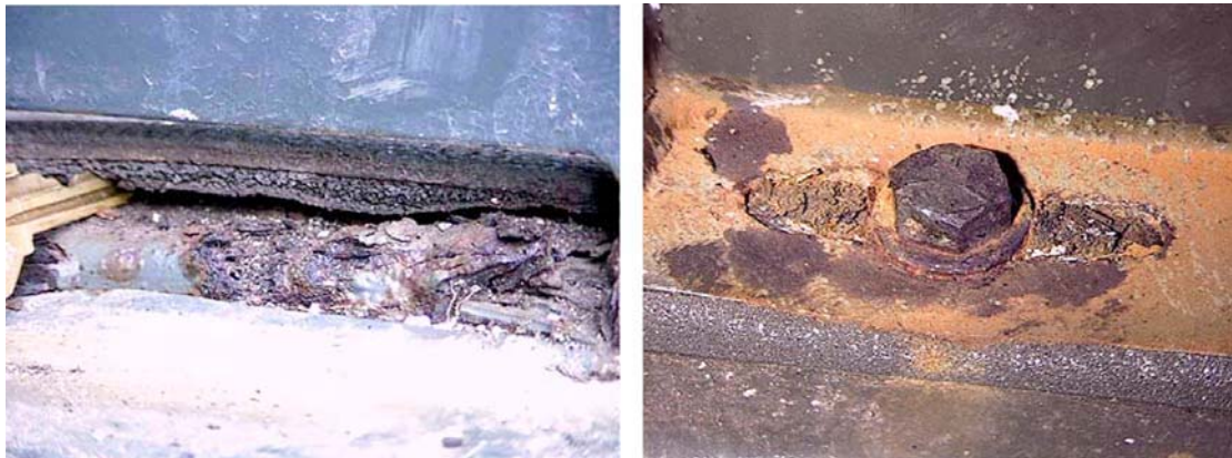
Figure 1-3. Open Cell Foam and Resulting Corrosion
