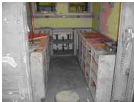
Figure 4-1. Electronic Shelter: Installed Wood Cabinetry
