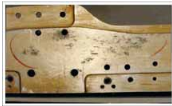
Figure 3-7. Pitting of an Aluminum Angle Assembly
