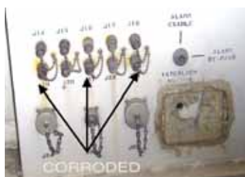
Figure 8-1. ANMST-TIV Corroded Exterior Plugs
