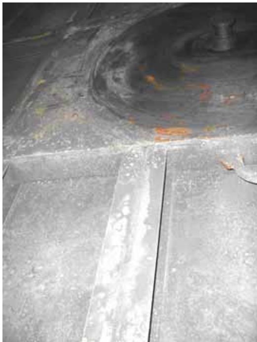
Figure 10-13. Corrosion Undercarriage of Shelter
