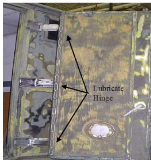
Figure 10-8. Electronic Shelter Door
