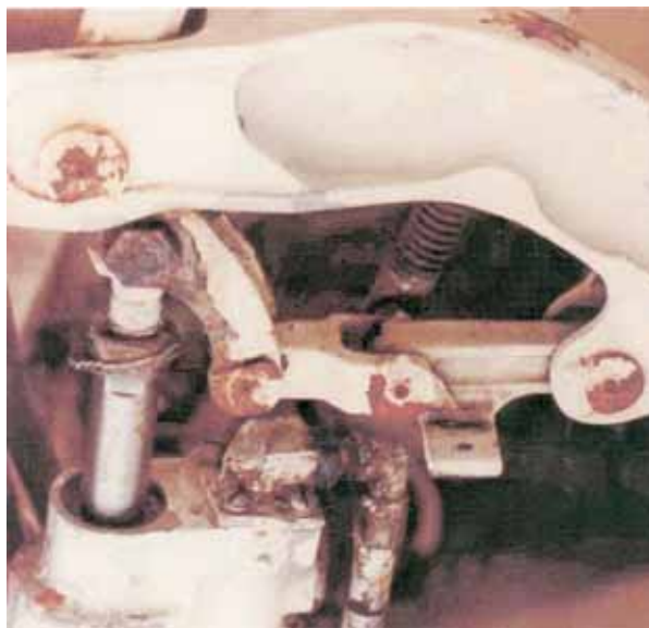
Figure 3-19. Steel Corrosion Products (Rust)
