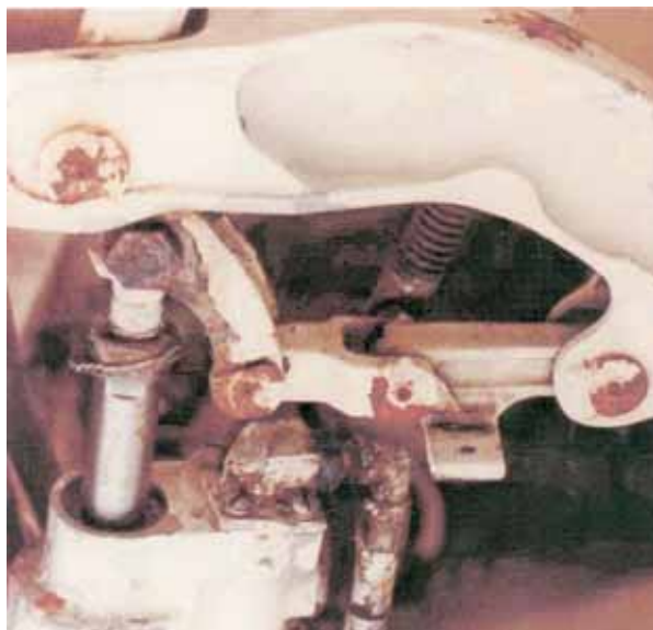
Figure 3-19. Steel Corrosion Products (Rust)
