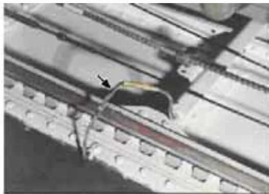
Figure 10-11. Bonding Cable Between Frame and Door
