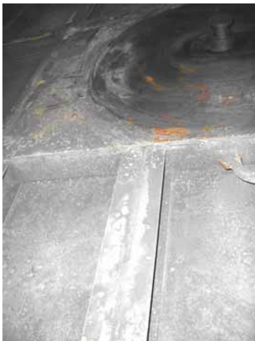
Figure 10-13. Corrosion Undercarriage of Shelter
