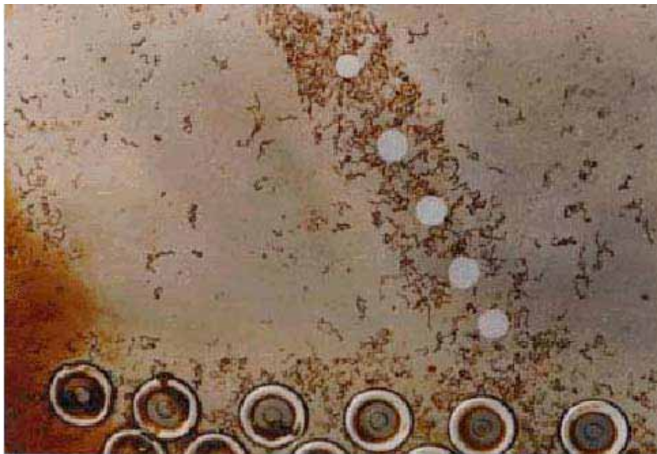
Figure 3-15. Filiform Corrosion Found Under a Paint Coating on a Magnesium Alloy Panel
