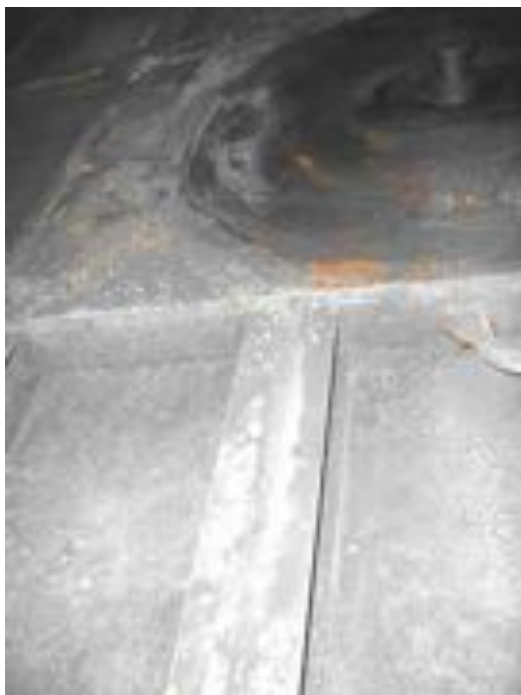
Figure 10-13. Corrosion Undercarriage of Shelter
