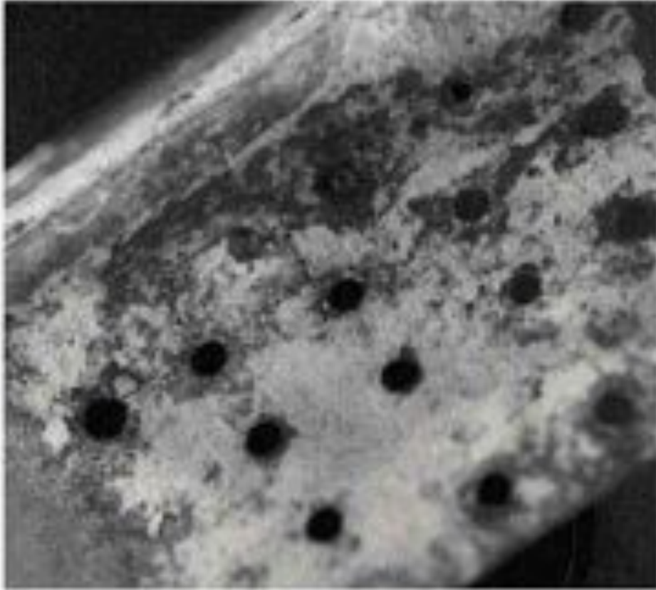
Figure 3-20. Aluminum Surface Corrosion Products
