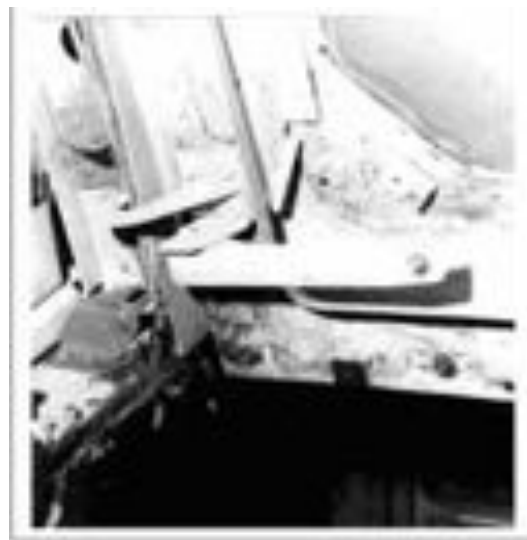
Figure 10-10. Corroded Battery Compartment
