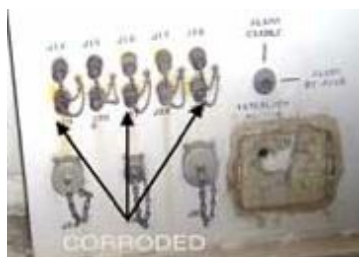
Figure 8-1. ANMST-TIV Corroded Exterior Plugs
