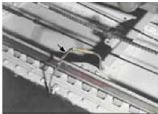
Figure 10-11. Bonding Cable Between Frame and Door
