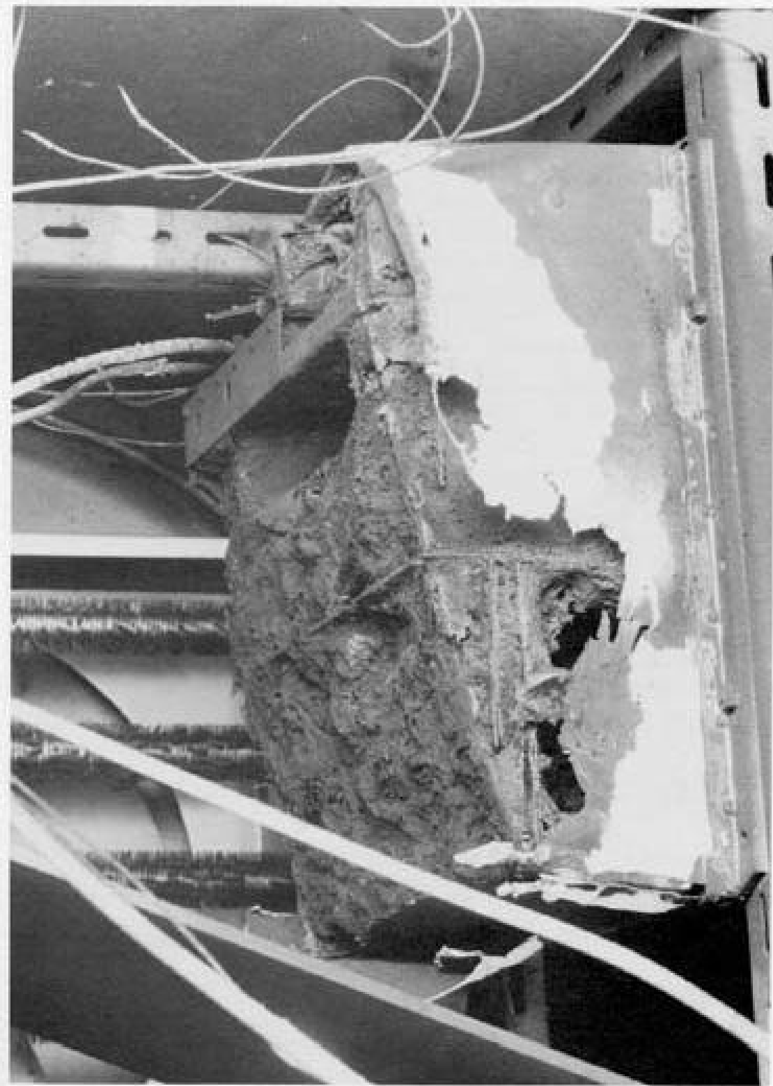
Figure 6-5 - Static inverter (post-test).
