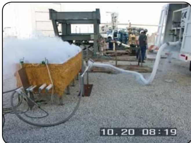
Ground support equipment designed at Kennedy Space Center is used to transfer cryogenic fluid. Condensation caused by the extremely cold fluid is visible in this image.
