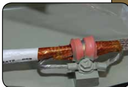
This close-up shows the final splicing completed on the wiring between space shuttle Atlantis' external tank and the engine cutoff (ECO) sensor system. Cryogenic shielding is installed around the wiring.
