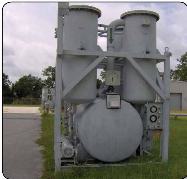
An oxidizer vapor scrubber is shown outside the Payload Hazardous Servicing Facility.
