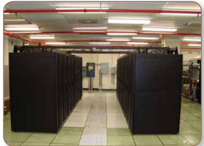
The Kennedy Data Center provides agency patchlink and reporting services.
