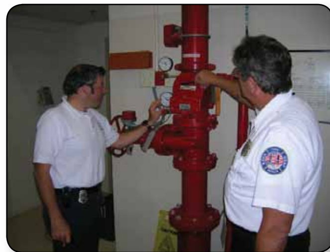
Kennedy Space Center engineers participate in fire protection activities.
