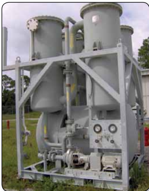
A fuel vapor scrubber is shown outside the Payload Hazardous Servicing Facility.
