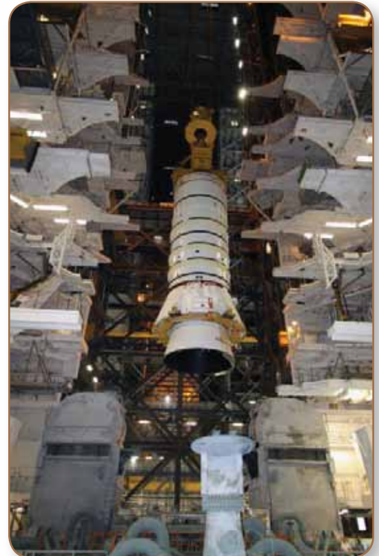
Workers carefully lift a solid rocket motor segment for the Ares I-X project.
