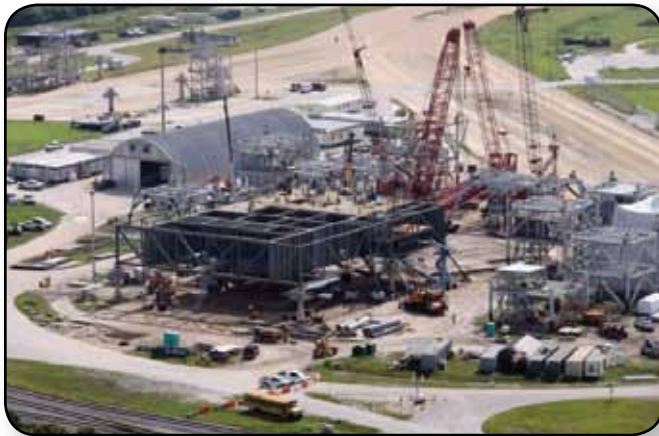
A new mobile launcher is built in the construction and refurbishment area at NASA's Kennedy Space Center in Florida.
