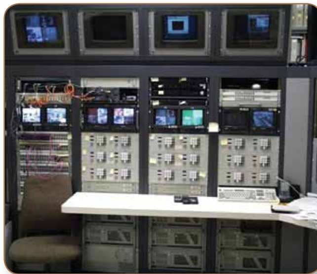
Equipment in the Telescience and Internet Systems Laboratories support video streaming over Internet Protocol (IP).
