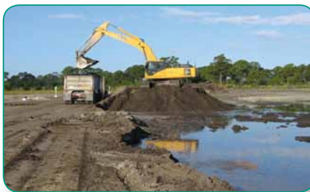
A hazardous waste soil excavation is performed at the Kennedy Athletic Recreation and Social (KARS) Park.
