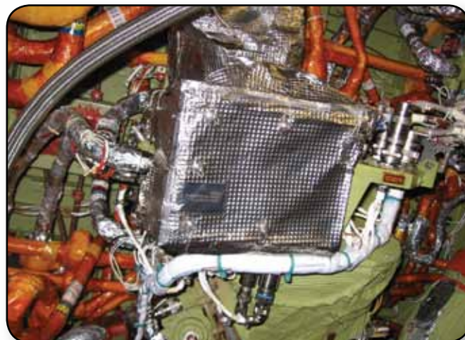
An assessment was performed to evaluate the risks of an electrostatic discharge from ungrounded metallic thermal blankets located in the aft compartment of the orbiter.
