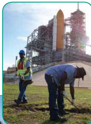
The Post Emergency Spill Cleanup Team removes contaminated soil from Launch Complex 39A.
