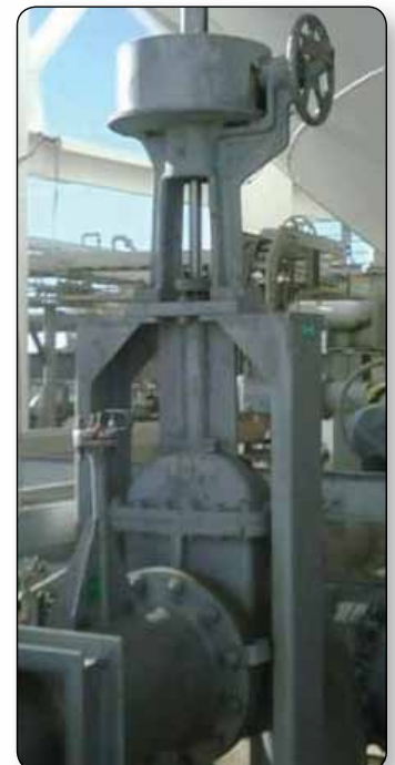
This cryogenic valve is part of an overall pressure system, one of many that KSC certifies.
