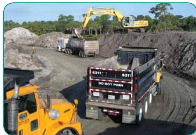
Excavation activities at the Kennedy Athletic Recreation and Social (KARS) Park resulted in the removal of more than 100,000 tons of contaminated soil.
