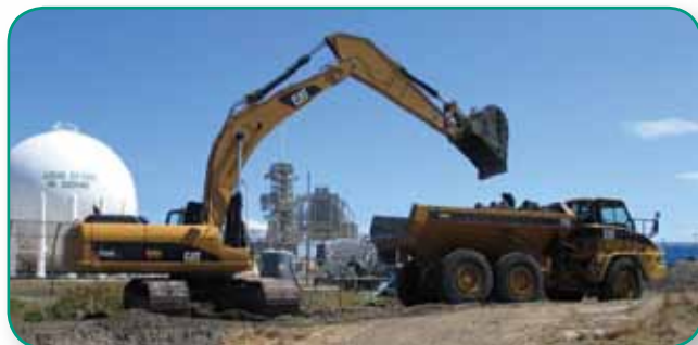
Excavation activities in the Launch Pad 39A area resulted in removal of a contaminated source area.
