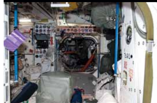
Interior of Node 1 looking in to Node 3.
