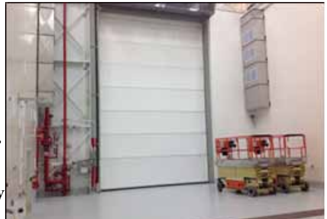
Figure 3-12. Inside Spacecraft Fueling Facility
