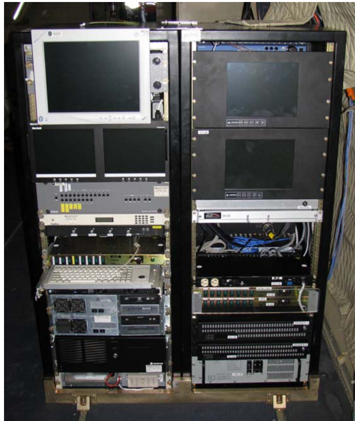
Figure 5-4. Project data system rack
