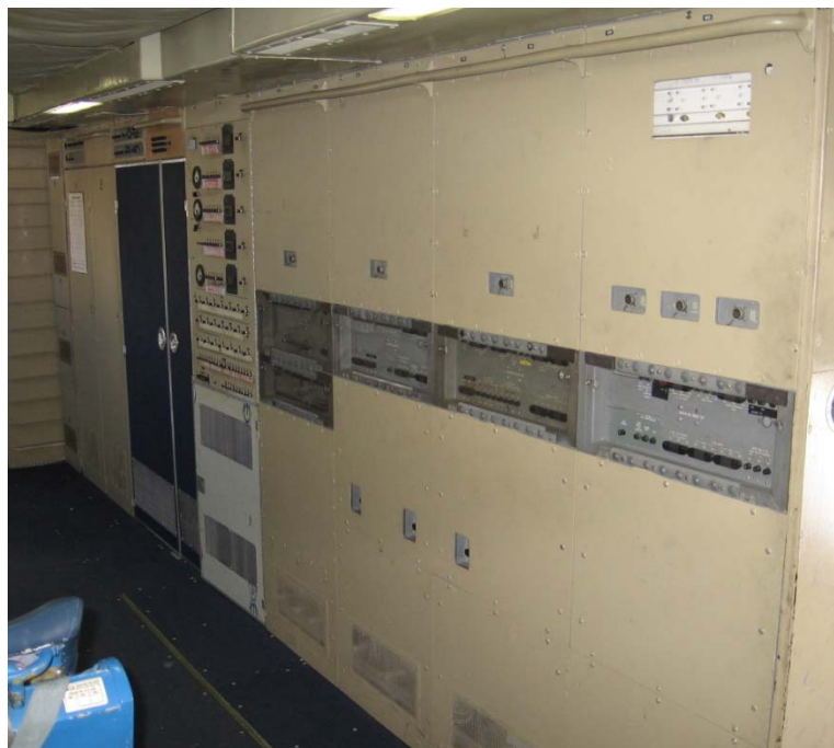
Figure 4-14. Electrical load center
