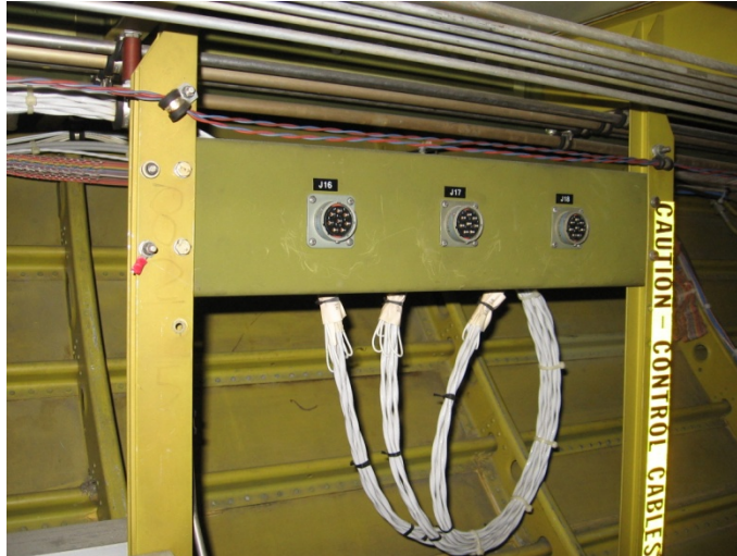
Figure 4-16. Power station below the cabin floor
