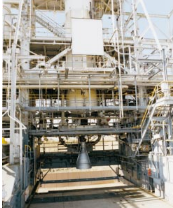
Figure 15-15: Close-up of the missile testing bay in Figure 15-14 showing the engine, feed lines, and run tanks.
