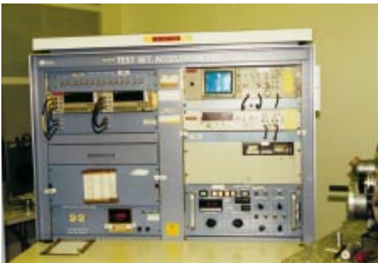
Figure 9-24: PIGA accelerometer alignment station control electronics.
