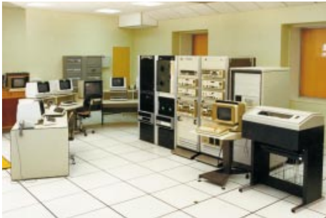
Figure 12-18: Representative ground-site telemetry receiving and processing equipment.
