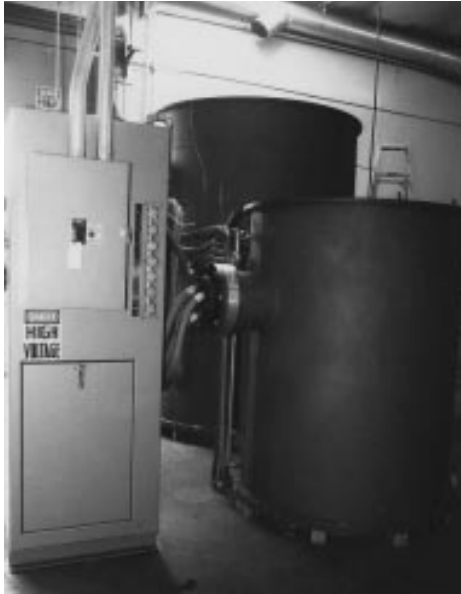
Figure 7-9: Two small CVD furnaces and an induction power supply.
