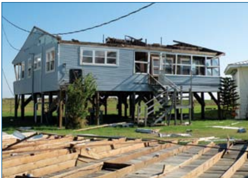
FIGURE 4-17: Roof structure that was poorly connected to the house (Jefferson Parish, LA) (SOURCE: FEMA P-757)
