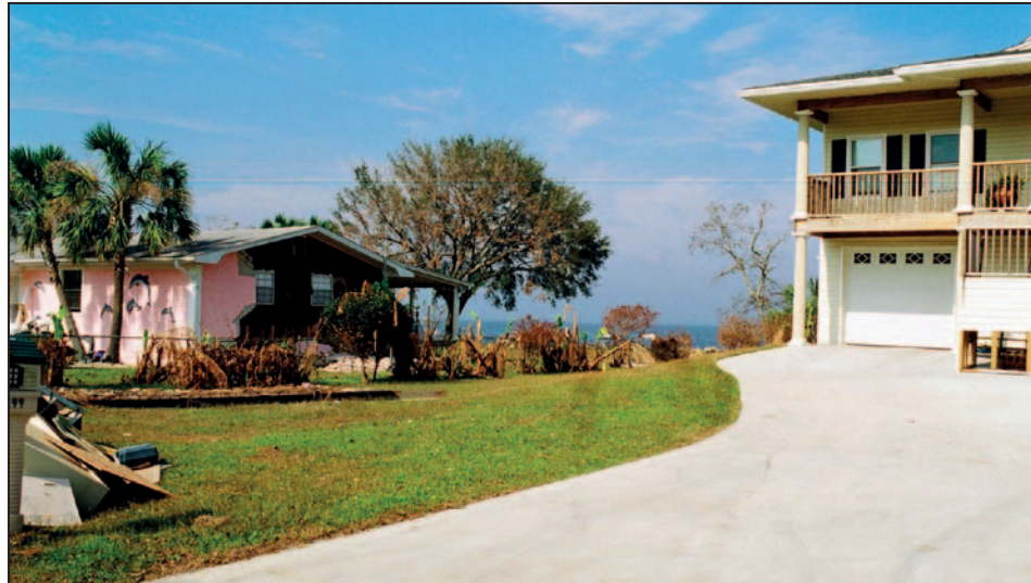
Figure 2-15. The pre-FIRM house (left) experienced damage due to surge and waves while the newer, elevated, post-FIRM house (right) experienced minimal damage, Hurricane Ivan (Santa Marina, Pensacola, FL, 2005)
