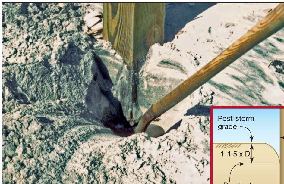
Figure 3-48. Determination of localized scour from changes in sand color, texture, and bedding (Hurricane Fran, 1996)
