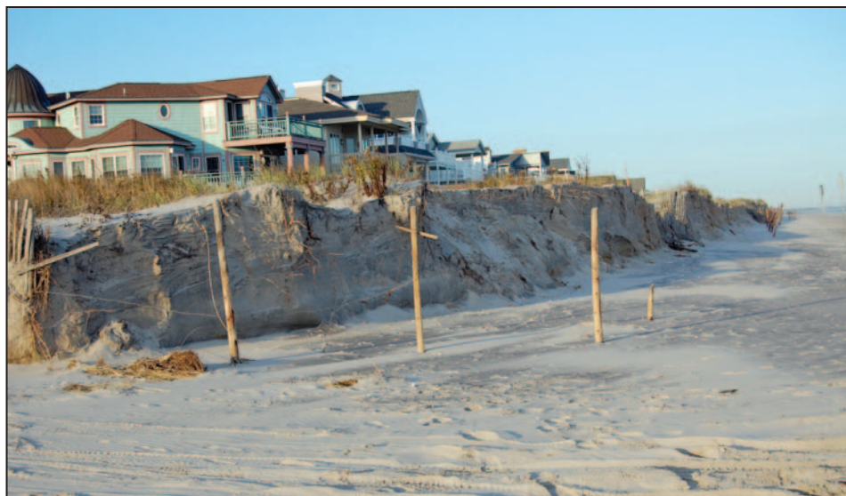
Figure 3-31. Dune erosion in Ocean City, NJ, caused by the remnants of Hurricane Ida (2009) and a previous nor'easter
