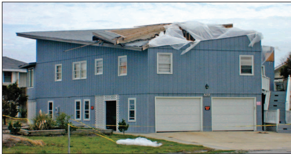
Figure 4-4. Although sited away from the shore, winds from Hurricane Floyd (1999) tore off the large overhanging roof of this house in Wrightsville Beach, NC
