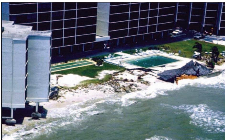
Figure 4-24. Beach erosion and damage due to a destroyed bulkhead at Bonita Beach, FL, from a subtropical storm
