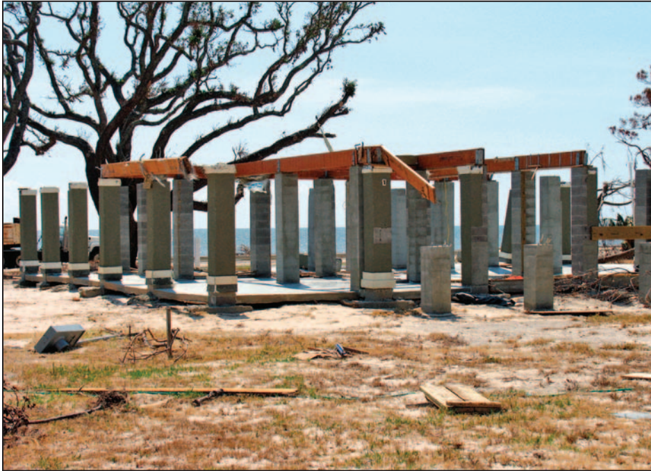
Figure 2-5. This elevated house atop a masonry pier foundation was lost, probably due to waves and storm surge reaching above the top of the foundation, Hurricane Katrina (Long Beach, MS, 2005)
