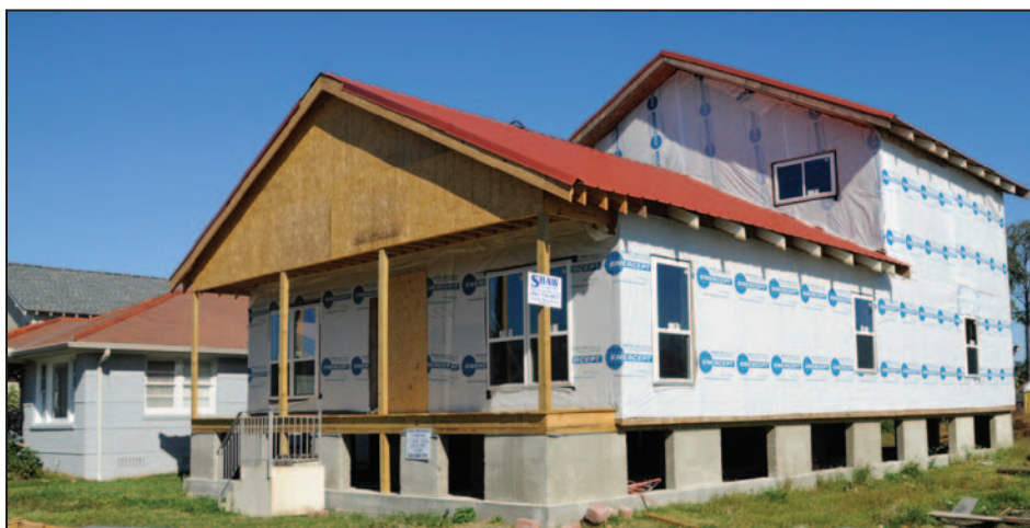
Figure 4-2. Redevelopment on a previously developed lot as part of the rebuilding process after Hurricane Katrina (Lakeview, LA)
