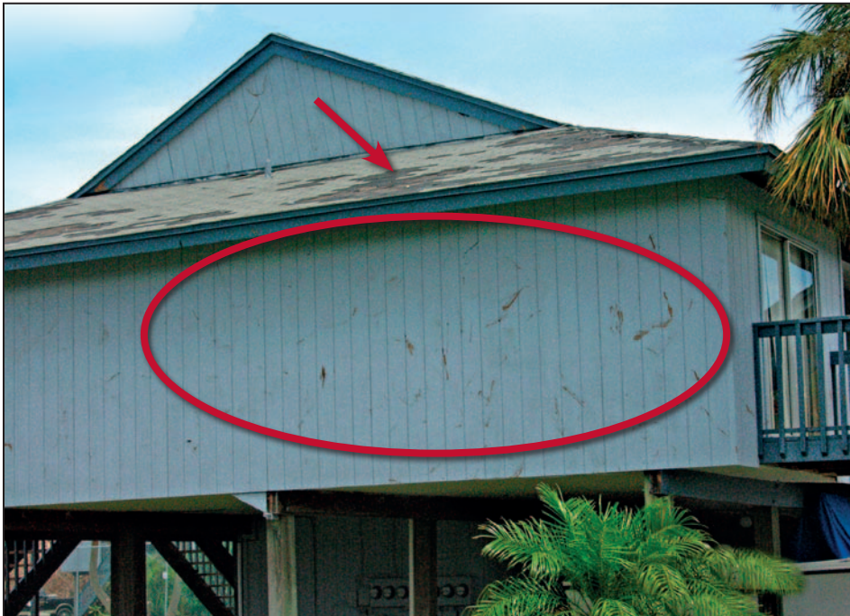
Figure 11-2. Numerous wind-borne debris scars on the wall of this house and several missing asphalt shingles. Estimated wind speed: 140 to 150 mph. Hurricane Charley (Florida, 2004)
