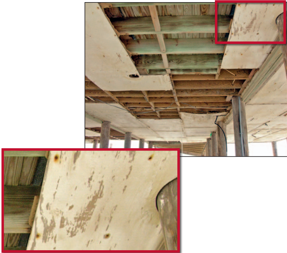
Figure 11-4. Plywood panels on the underside of a house that blew away because of excessive nail spacing. Note the corroded nails (inset). Estimated wind speed: 105 to 115 mph. Hurricane Ivan (Alabama, 2004)
