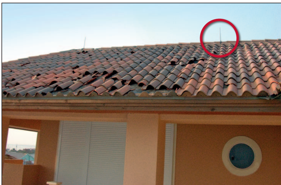
Figure 11-48. The fastener heads on this mechanically attached tile roof had corroded; air terminals (lightning rods) in a lightning protection system (circle). Hurricane Ivan (Alabama, 2004)
