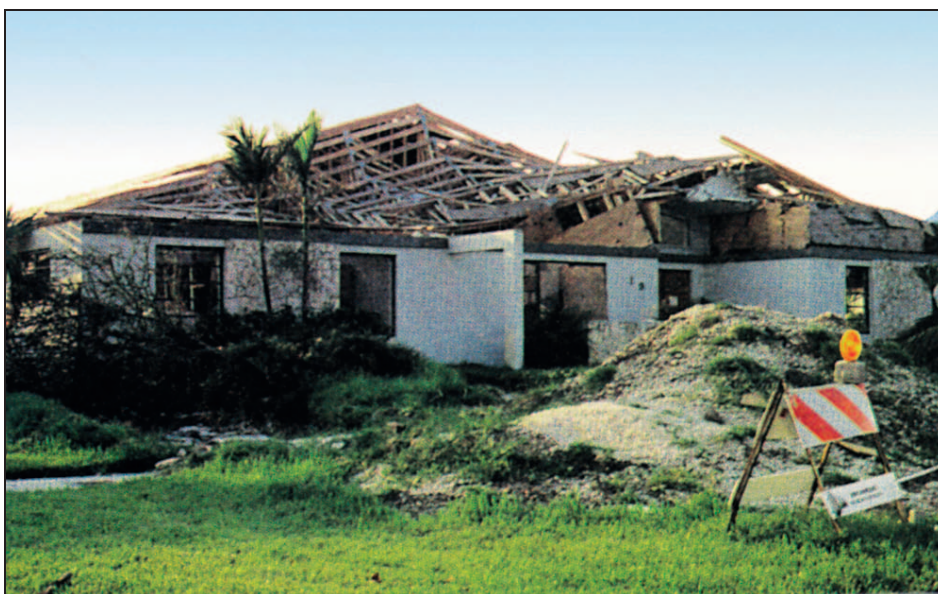
Figure 9-21. Gable-end failure, Hurricane Andrew (Dade County, FL, 1992)
