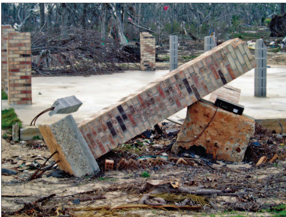
Figure 10-17. Performance comparison of pier foundations: piers on discrete footings (foreground) failed by rotating and overturning while piers on more substantial footings (in this case a concrete mat) survived Hurricane Katrina (Pass Christian, MS, 2005)
