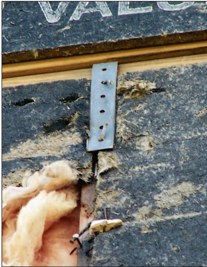
Figure 13-15. Connector failure caused by insufficient nailing
