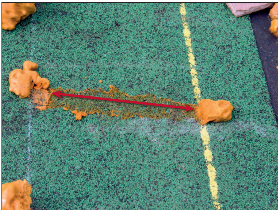
Figure 11-44. Adhesive that debonded from the cap sheet
