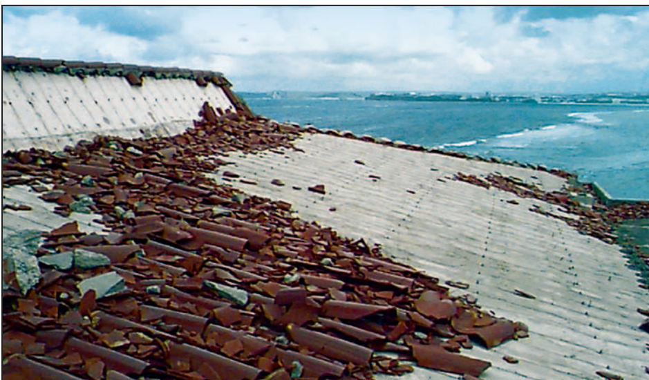
Figure 11-41. Blow-off of wire-tied tiles installed over a concrete deck. Typhoon Paka (Guam, 1997)
