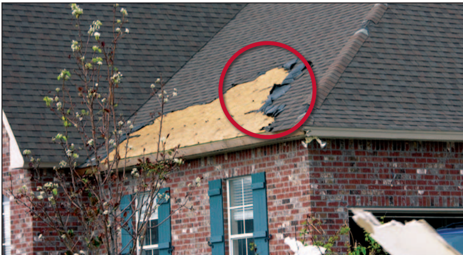
Figure 11-30. Loss of shingles and underlayment along the eave and loss of a few hip shingles. Estimated wind speed: 115 mph. Hurricane Katrina (Louisiana, 2005)
