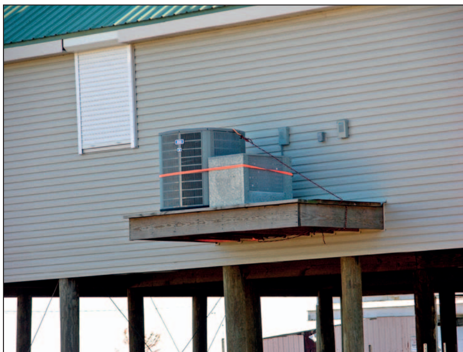
Figure 12-2. Proper elevation of an air-conditioning condenser in a floodprone area; additional anchorage is recommended
