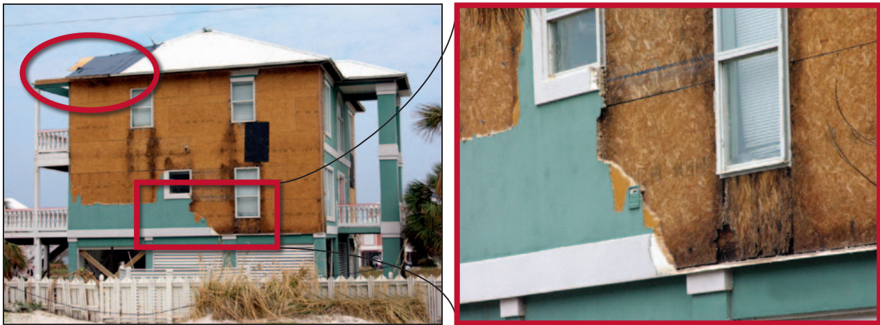
Figure 11-21. EIFS with a barrier design: blown-off roof decking (top circle); severely rotted OSB due to leakage at windows (inset). Hurricane Ivan (2004)
