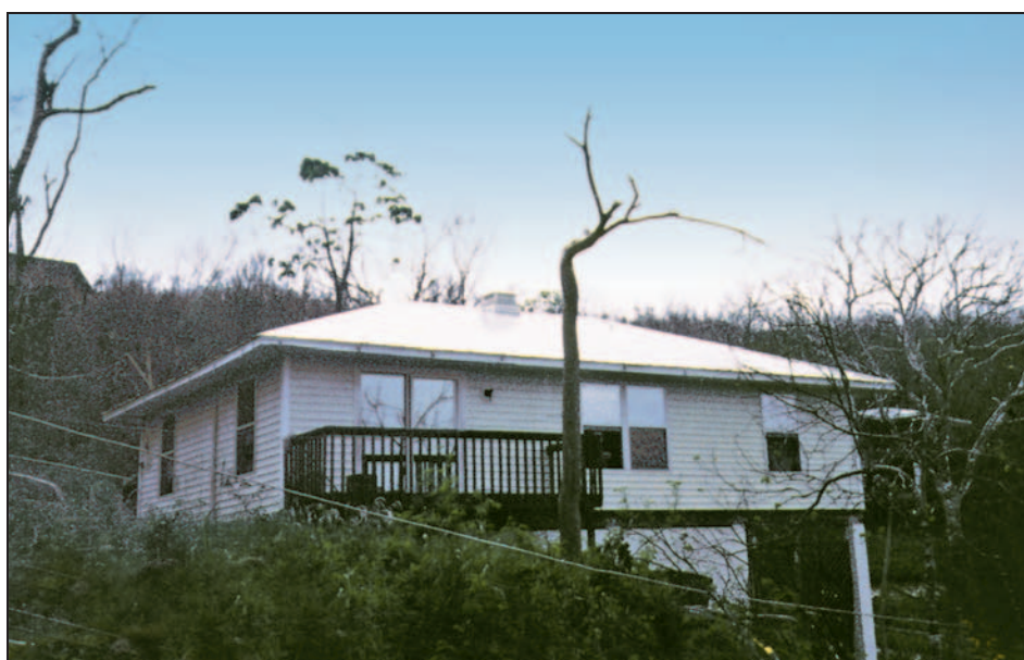
Figure 9-27. Hip roof that survived high winds with little to no damage, Hurricane Marilyn (U.S. Virgin Islands, 1995)
