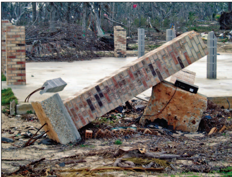
Figure 10-17. Performance comparison of pier foundations: piers on discrete footings (foreground) failed by rotating and overturning while piers on more substantial footings (in this case a concrete mat) survived Hurricane Katrina (Pass Christian, MS, 2005)
