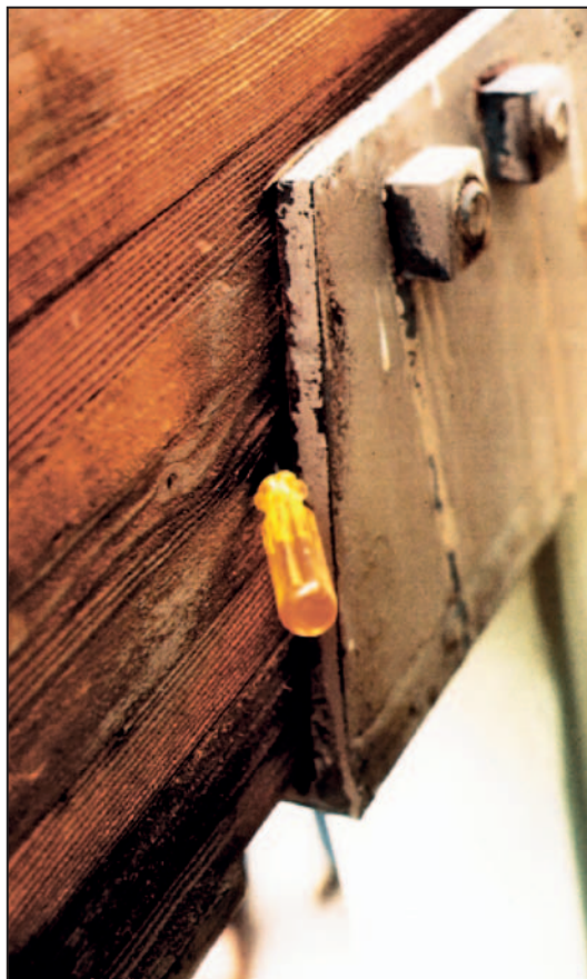
Figure 14-2. Wood decay behind a metal beam connector
