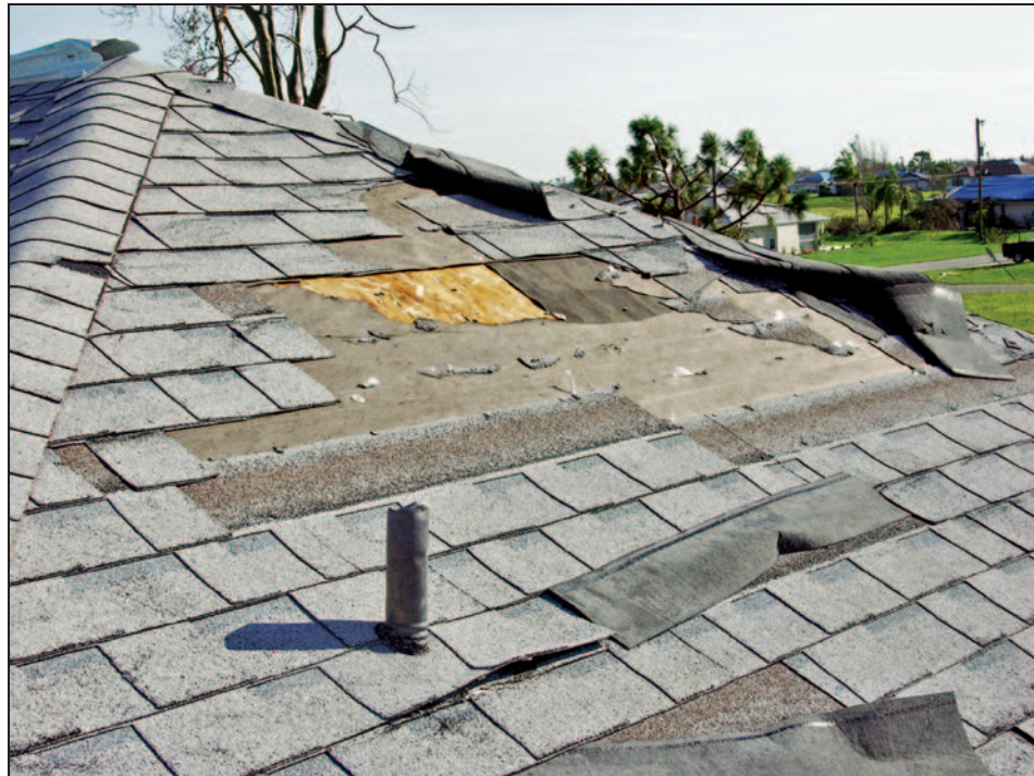
Figure 11-24. Small area of sheathing that was exposed after loss of a few shingles and some underlayment. Estimated wind speed: 140 to 160 mph. Hurricane Charley (Florida, 2004)
