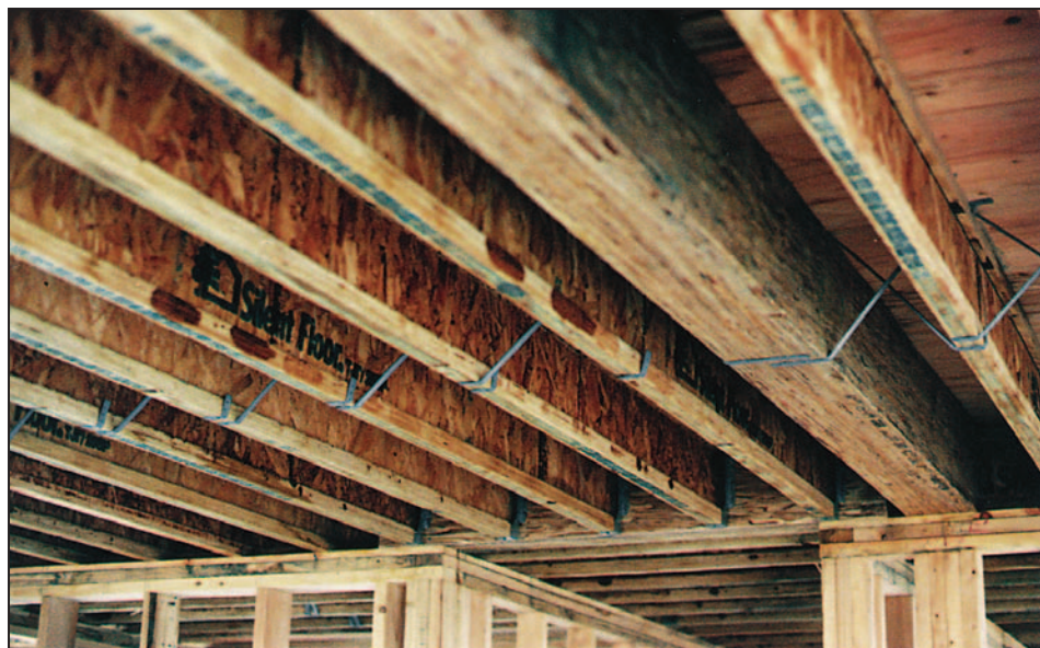
Figure 13-20. Engineered joists used as floor joists with proper metal brace to keep the bottoms of the joists from twisting; engineered wood beam
