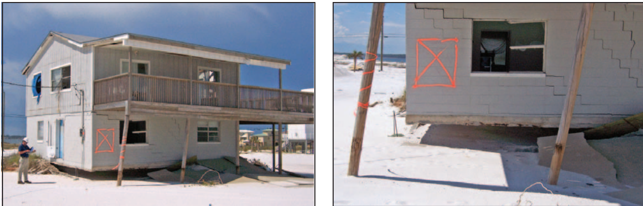
Figure 10-1. Closed foundation failure due to erosion and scour undermining; photograph on right shows a close-up view of the foundation failure and damaged house wall, Hurricane Dennis (Navarre Beach, FL, 2005)
