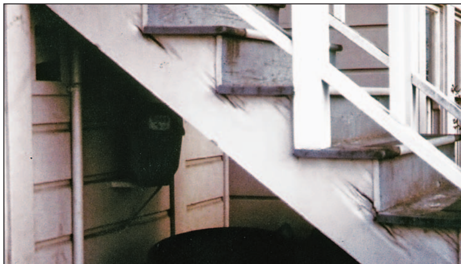
Figure 13-13. Deterioration in a notched stair stringer
