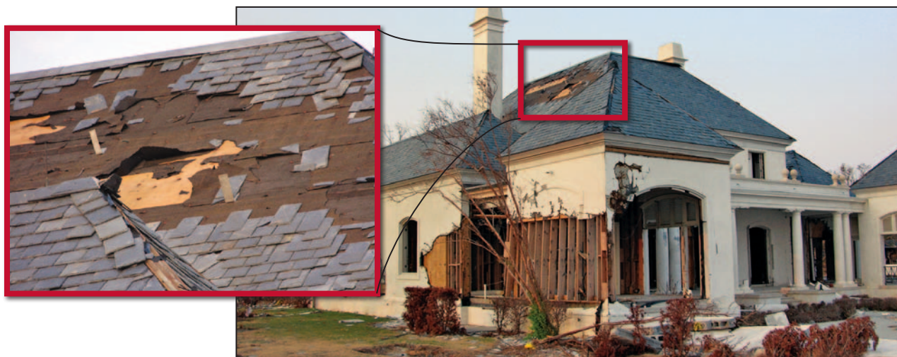
Figure 11-53. Damaged slate roof with nails that typically pulled out of the deck. Some of the slate broke and small portions remained nailed to the deck. Estimated wind speed: 130 mph. Hurricane Katrina (Mississippi, 2005)
