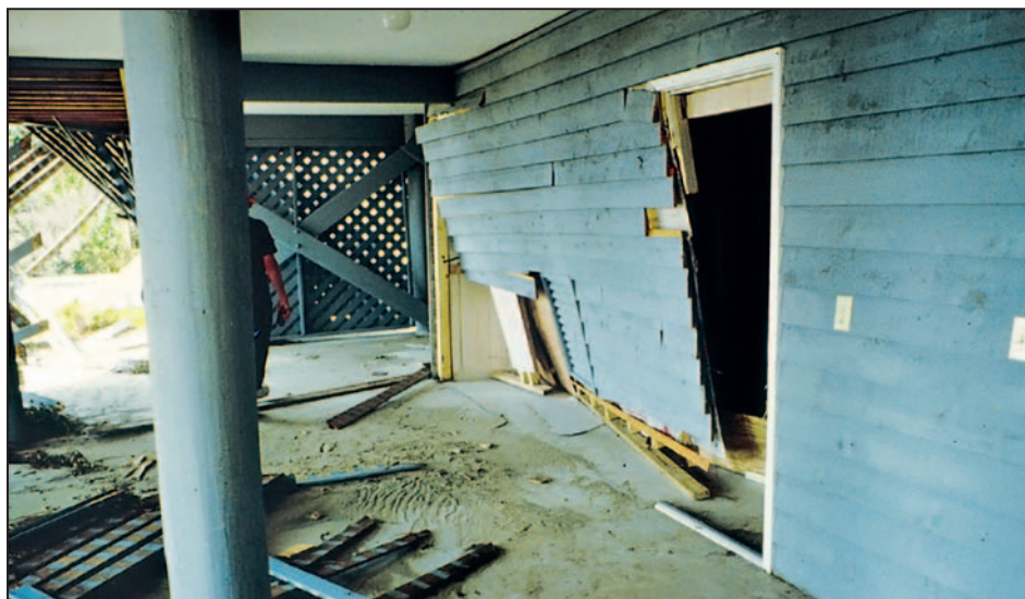
Figure 9-28. Typical failure mode of breakaway wall beneath an elevated building—failure of the connection between the bottom plate of the wall and the floor of the enclosed area, Hurricane Hugo (South Carolina, 1989)
