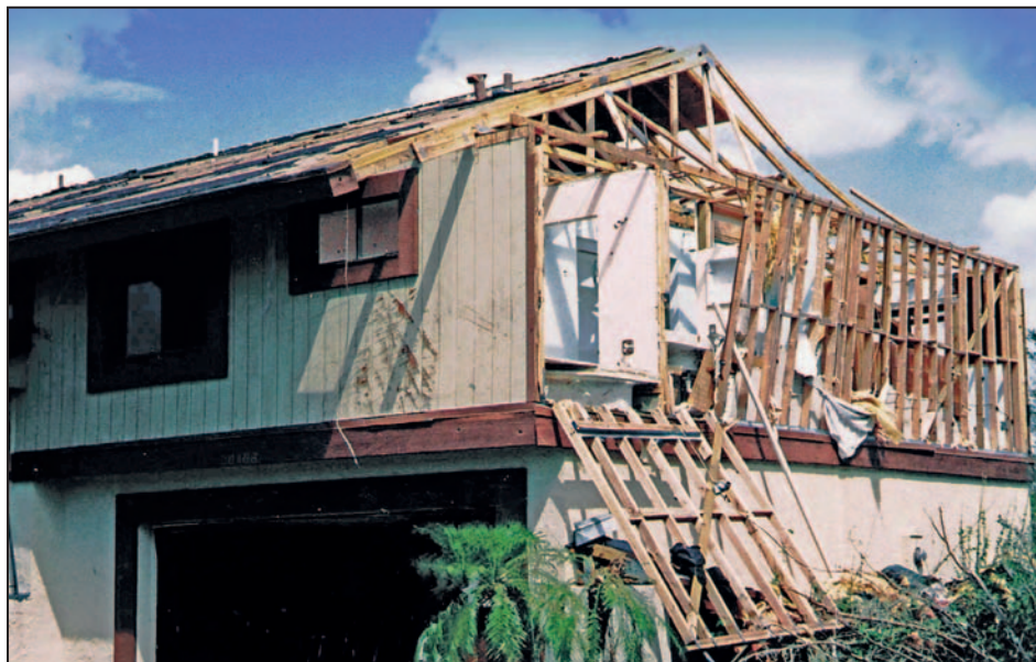
Figure 9-1. Load path failure at gable end, Hurricane Andrew (Dade County, FL, 1992)
