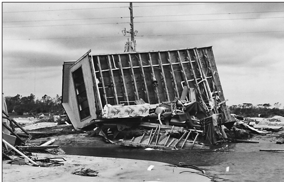
Figure 9-2. Load path failure in connection between home and its foundation, Hurricane Fran (North Carolina, 1996)
