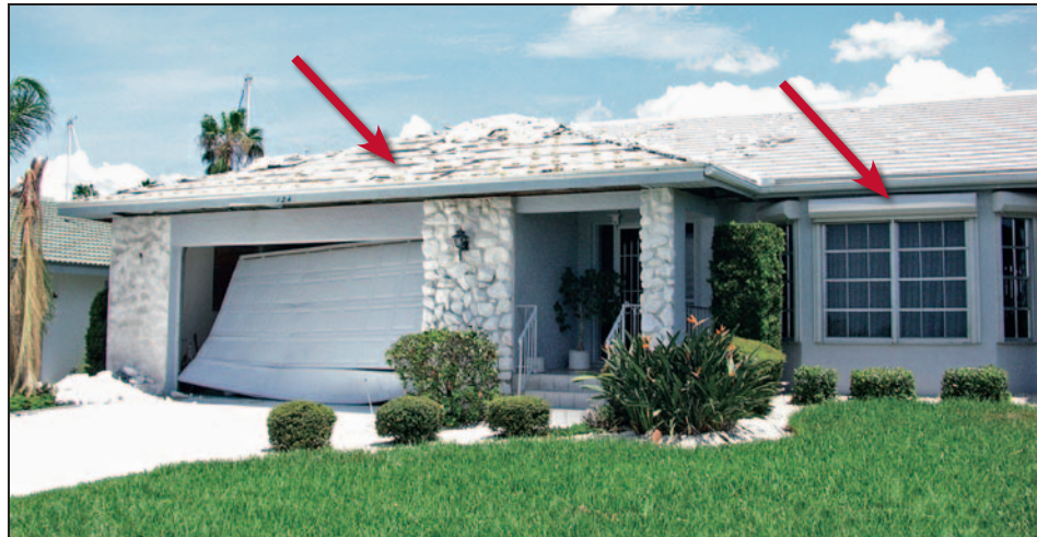
Figure 11-6. Garage door blown from its track as a result of positive pressure. Note the damage to the adhesive-set tiles (left arrow; see Section 11.5.4.1). This house was equipped with roll-up shutters (right arrow; see Section 11.3.1.2). Estimated wind speed: 140 to 160 mph. Hurricane Charley (Florida, 2004)
