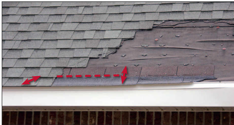
Figure 11-32. Incorrect installation of the starter course (incorrectly rotated starter, right arrow, resulted in self-seal adhesive not near the eave, dashed line). Estimated wind speed: 130 mph. Hurricane Katrina (Mississippi, 2005)
