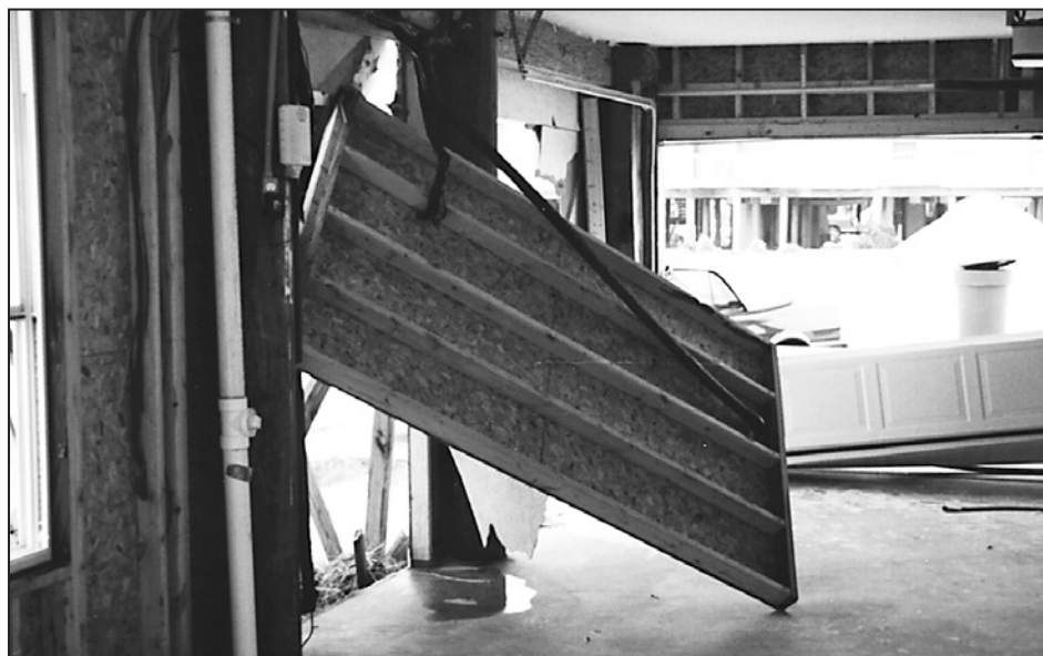
Figure 9-29. Breakaway wall panel prevented from breaking away cleanly by utility penetrations, Hurricane Opal (Florida, 1995)
