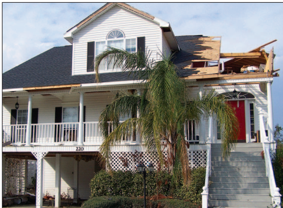
Figure 9-5. Newer home damaged from internal pressurization and inadequate connections, Hurricane Katrina (Pass Christian, MS, 2005)
