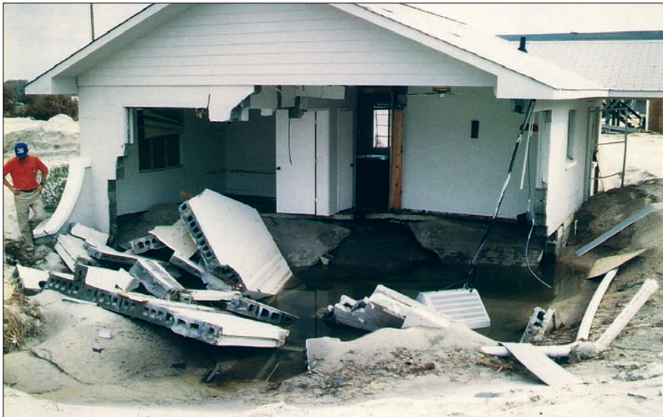
Figure 1-13. Extreme case of localized scour undermining a slab-on-grade house in Topsail Island, North Carolina, after Hurricane Fran (1996). Prior to the storm, the lot was several hundred feet from the shoreline and mapped as an A zone on the FIRM. This case illustrates the need for open foundations in Coastal A zones.
