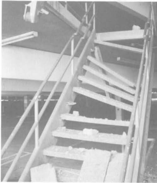
Earthquake Damage: 1994, Northridge, California Photo Credit: Wiss, Janney, Elstner Associates, Inc.
