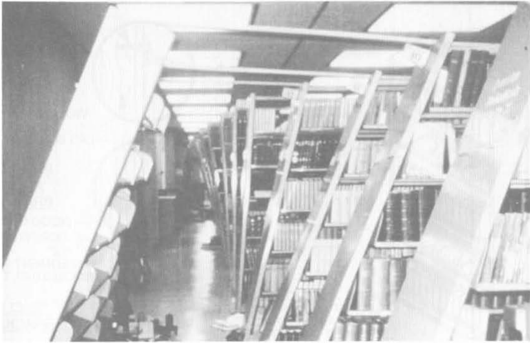
Failure of inadequately upgraded library shelving Earthquake Damage: 1987, Whittier Narrows, California Photo Credit: Earthquake Engineering Research Institute, Marshall Lew & Greg Brandow C12b
