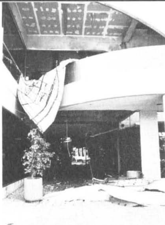
Failure of heavy stucco soffit at building entrance Earthquake Damage: 1994, Northridge, California Photo Credit: Robert Reitherman
