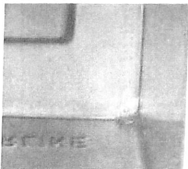
6-K. Permissible Excessive Paint, Interior
