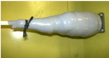
Acceptable Dual wrap kit installed properly using self-leveling green, stretch seal (inner, pink layer) and self-fusing silicone tape (outer, gray layer), secured with lacing tape.
