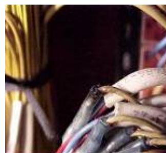
Unacceptable Overheating seen at the splice termination.
