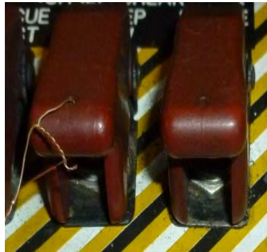
Unacceptable Shearwire not installed (right) and broken (left)
