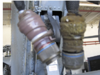
Unacceptable Self-fusing silicone tape not applied and not secured with authorized lacing tape.
