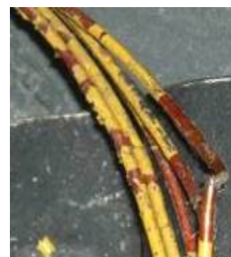
Unacceptable One wire shows exposed conductor; repair required
