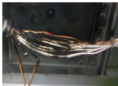
Unacceptable Wire bundle with more than 6 wires showing insulation overheat damage
