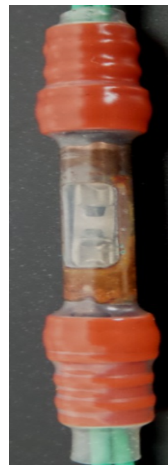
Unacceptable Evidence of corrosion inside sleeve. Multiple wires installed, both ends.
