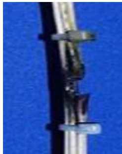
Unacceptable Arc tracking
