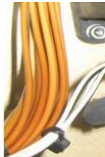
Unacceptable Overheating seen as a discoloration of the insulation (brown) compared to the white insulated wire.
