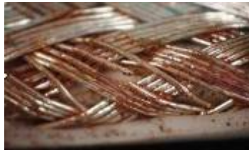
Unacceptable Broken strands and signs of corrosion on conductor/shielding.
