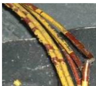
Unacceptable Polyimide/Kapton insulation removed, exposed bare conductor. Damaged wire section requires repair or replacement.
