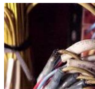
Unacceptable Overheating seen at the splice termination.
