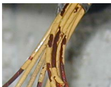
Acceptable Polyimide/Kapton insulation topcoat flaking shows degradation, but serviceable since no bare conductor exposed.
