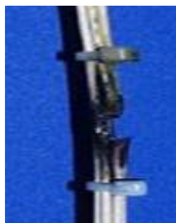
Unacceptable Arc tracking
