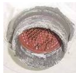
Unacceptable Another example of corrosion on a connector.
