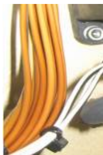
Unacceptable Overheating seen as a discoloration of the insulation (brown) compared to the white insulated wire.
