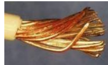
Unacceptable Severe corrosion on wire conductor.
