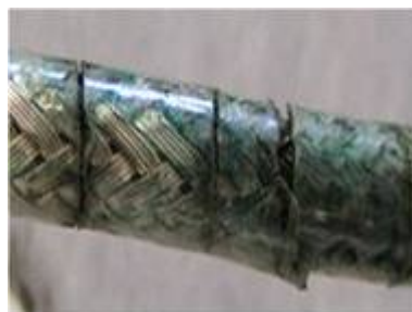
Unacceptable Radial crack in the insulation.
