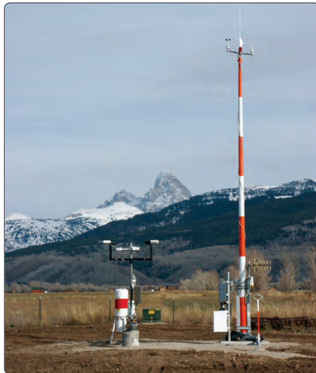
Figure 1-11. AWSS installation at Driggs-Reed, Idaho.
