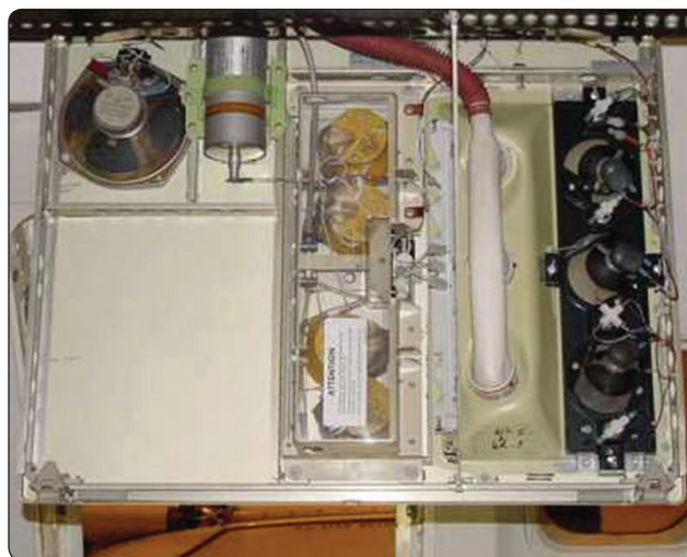
Figure 16-29. An oxygen generator mounted in place in an overhead passenger service unit of an air transport category aircraft.
