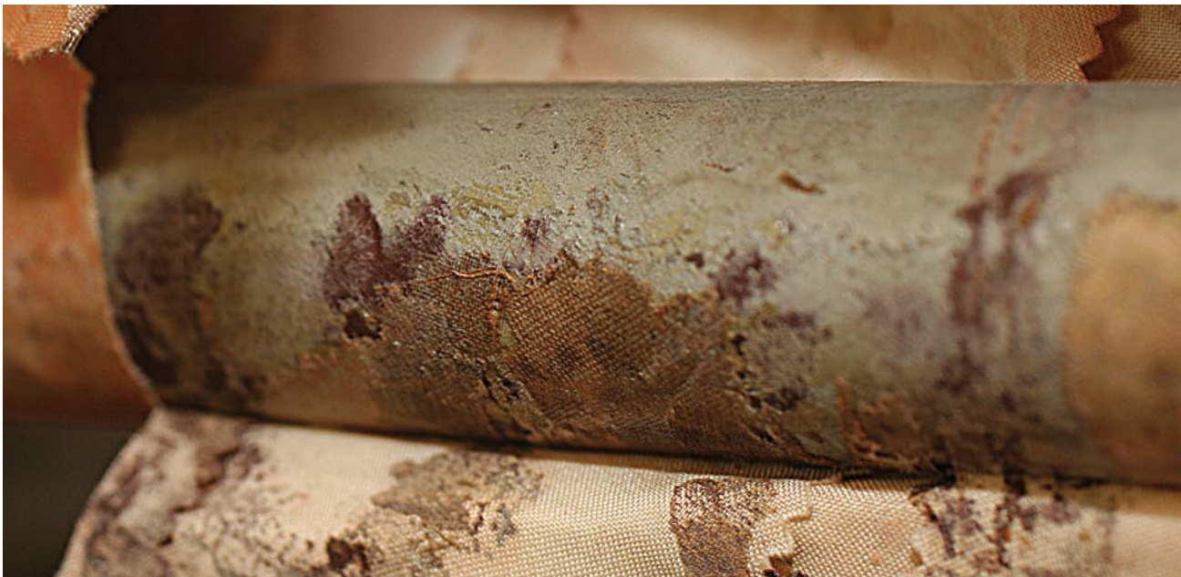
Figure 6-15. Rust on structural components.
