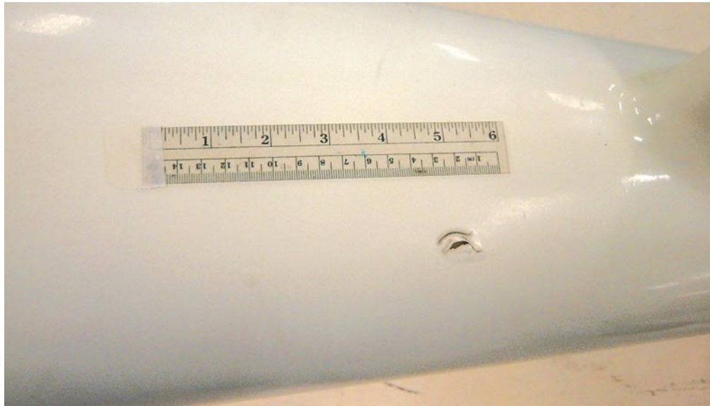
Figure 2-32. Digital image of impact damage.
