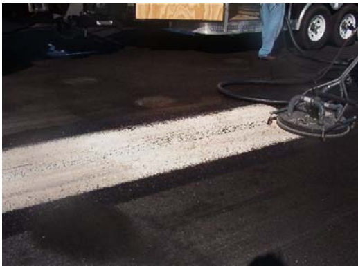
FIGURE 4-34. THE PROCESS USED TO REMOVE OIL STAIN.
