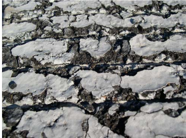
FIGURE 5-23. EVIDENCE OF BOTH PAINT AND ASPHALT CRACKING INDICATES PRE-EXISTING CONDITION.
