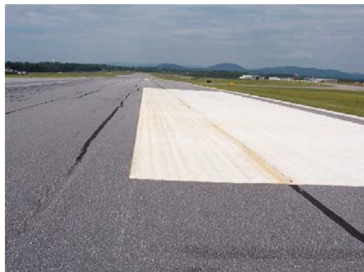
FIGURE 6-13. JOINT MATERIAL DISCOLORS THE WHITE PAINT.
