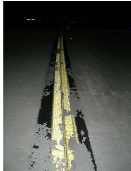
FIGURE 4-8. EXAMPLE OF POOR REMOVAL OF CURING COMPOUND.
