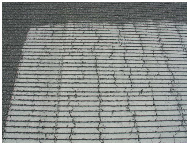
FIGURE 6-12. THE HEAVIER PAINT IN THE OVERLAP AREA CAUSED THE PAINT AND THE ASPHALT TO CRACK.
