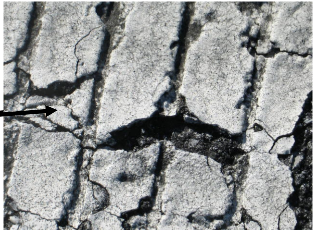
FIGURE 5-5. MAGNIFICATION OF CRACKED MARKINGS AND ASPHALT FROM FIGURE 5-4.
