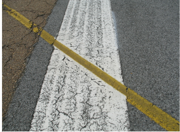
FIGURE 5-3. CRACKED AND PEELING MARKINGS – REMOVE 85 PERCENT.
