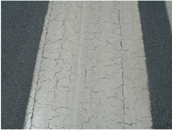
FIGURE 4-6. THIS MARKING IS 30 MONTHS OLD AND CRACKED.
