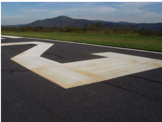
FIGURE 4-29. REPAINTING WITHOUT CLEANING THE STAIN RESULTS IN BLEED-THROUGH.
