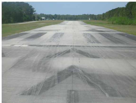
FIGURE 4-13. MARKINGS ARE OBSCURED BY ALGAE.
