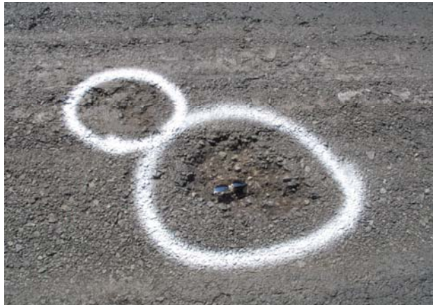
FIGURE 5-24. PRE-EXISTING CONDITION CAUSED BY OIL SPILL ON ASPHALT.
