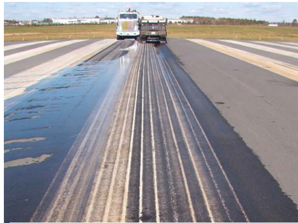
FIGURE 5-18. HIGH-PRESSURE WATERBLASTING IS EFFECTIVE FOR CLEANING LOOSE AND POORLY BONDED PAINT (SURFACE PREPARATION).
