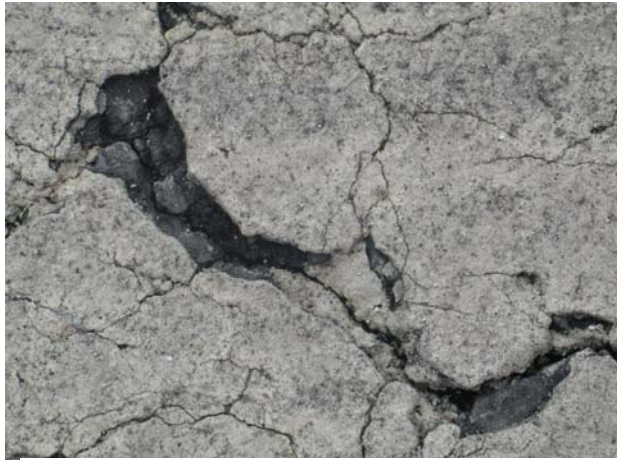
FIGURE 5-29. CRACKED PAINT INDICATES PRE-EXISTING PAVEMENT DETERIORATION.
