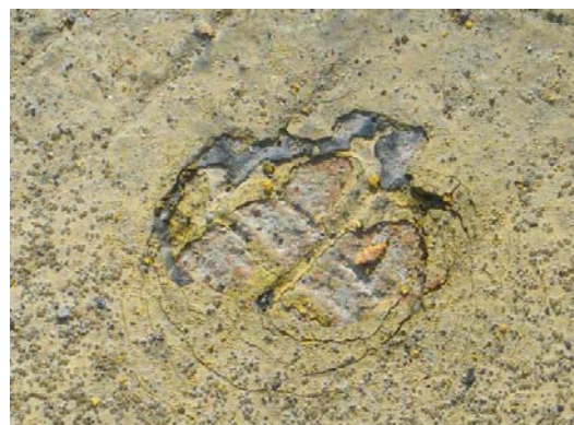
FIGURE 6-7. MULTIPLE LAYERS OF PAINT FILL THE GROOVES.
