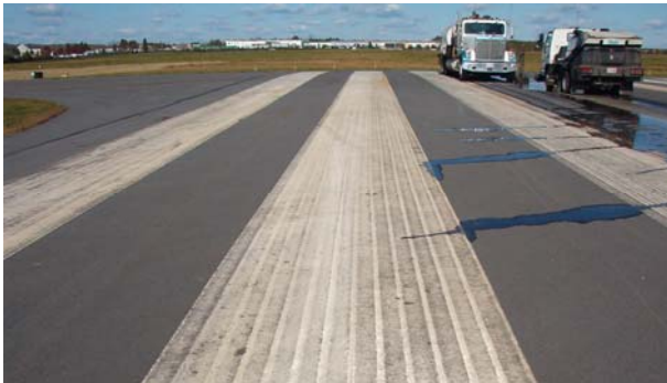
FIGURE 4-1. BEFORE CLEANING LOOSE AND POORLY BONDED PAINT.
