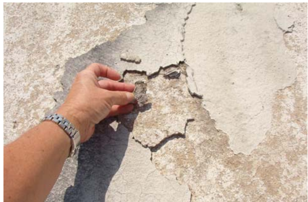
FIGURE 5-6. HEAVY PAINT BUILD UP ON CONCRETE.
