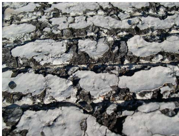
FIGURE 4-5. MAGNIFIED PHOTO OF FIGURE 4-4 SHOWS CRACKED ASPHALT WHERE WATER INVADES.
