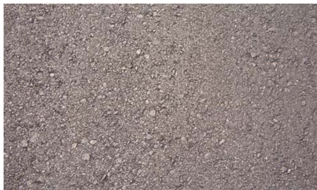
FIGURE 4-10. AFTER RUBBER REMOVAL.
