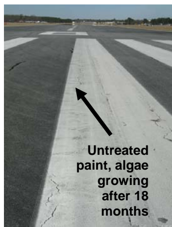
FIGURE 4-18. PAINT USED WAS STANDARD TT-P-1952E.
