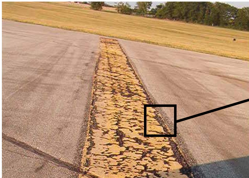
FIGURE 6-10. OLD SOLVENT PAINT CURLED, CRACKING THE ASPHALT TO WHICH IT WAS BONDED.
