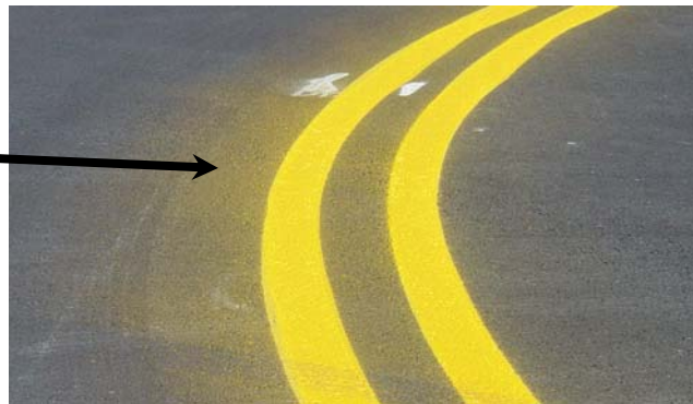
FIGURE 6-45. CLOSE UP OF OVER SPRAY IN FIGURE 6-44.
