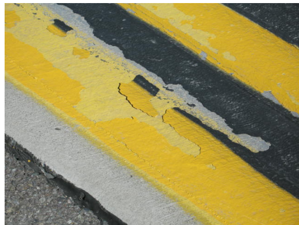
FIGURE 2-1. PEELING PAINT LAYERS
