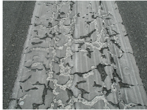
FIGURE 4-7. MANY LAYERS OF PAINT ON ASPHALT.
