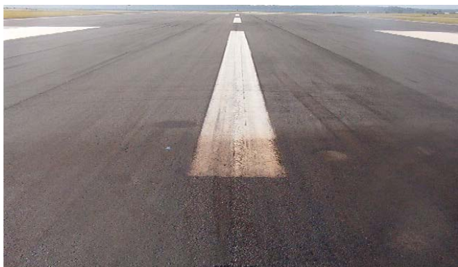
FIGURE 4-32. THE OILY STAIN WILL PREVENT NEW COATING FROM BONDING.
