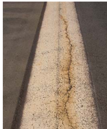
FIGURE 4-27. EVIDENCE OF RUST CONTAMINATION FROM SUBSTRATE.
