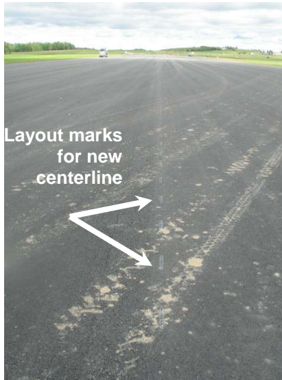
FIGURE 6-2. CONSTRUCTION DIRT MUST BE CLEANED.
