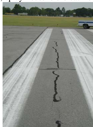
FIGURE 4-15. THE SAME SIDELINE AND THRESHOLD MARKING EIGHTEEN MONTHS LATER.
