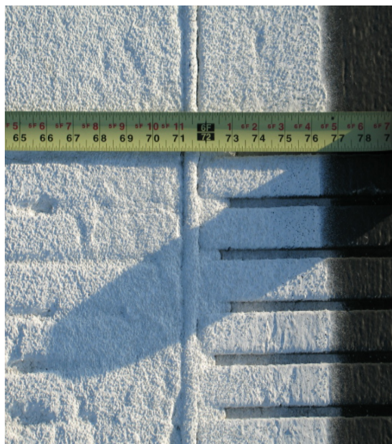
FIGURE 2-3. MARKING DIMENSION IS OUT OF TOLERANCE.
