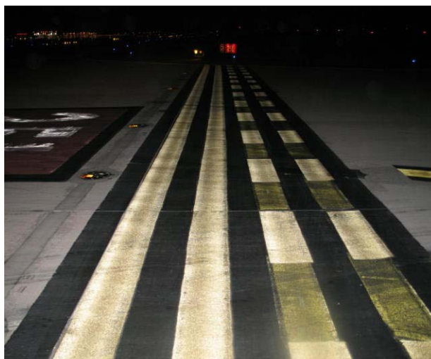
FIGURE 5-2. BLACK PAINT WEARS OFF, AND THE UNDERLYING COATING SHOWS THROUGH.
