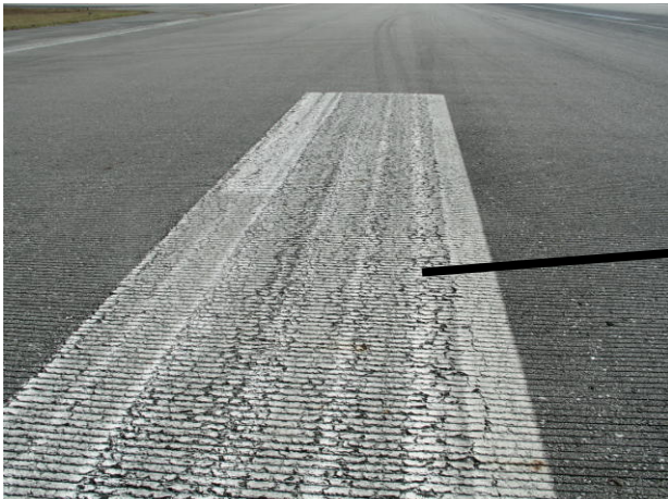
FIGURE 5-4. CRACKED MARKINGS WITH DETERIORATED ASPHALT UNDERNEATH IS A PRE-EXISTING CONDITION.
