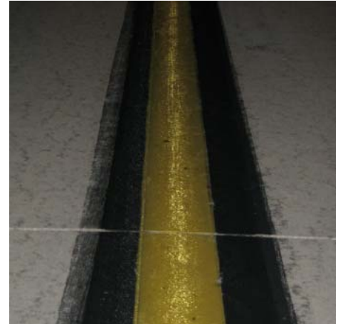
FIGURE 3-9. NON-FUNCTIONAL MARKING DUE TO POOR REFLECTIVITY.
