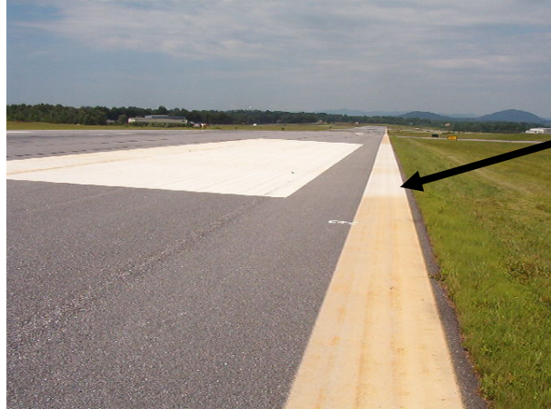
FIGURE 4-25. GROOVED SURFACE MAKES STAIN LESS NOTICEABLE.
