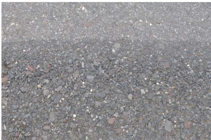
FIGURE 5-25. REMOVAL OF MARKINGS FROM NEW ASPHALT RESULTS IN EXPOSED AGGREGATE (SCARRING).
