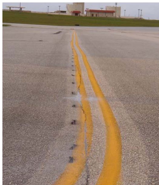
FIGURE 2-4. MARKING IS OUT OF ALIGNMENT
