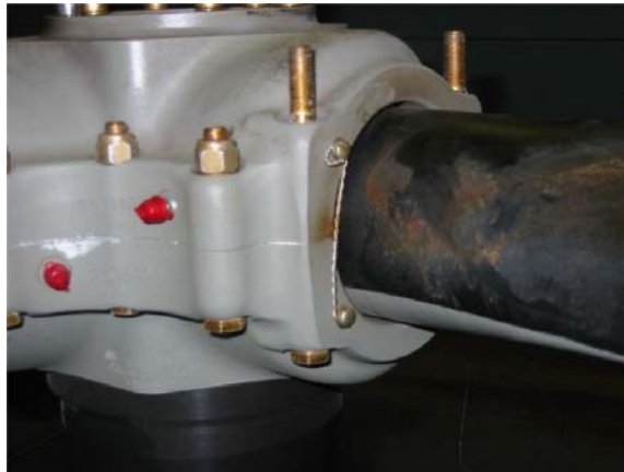
FIGURE 2-1. Grease Leak Residues
