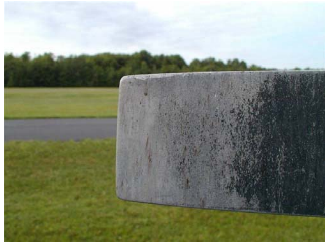
FIGURE 1-7. Erosion on a Metal Blade
