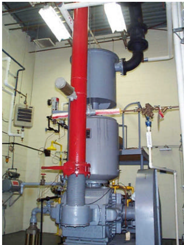
PHOTO 6 Vacuum for Decompression Chamber
