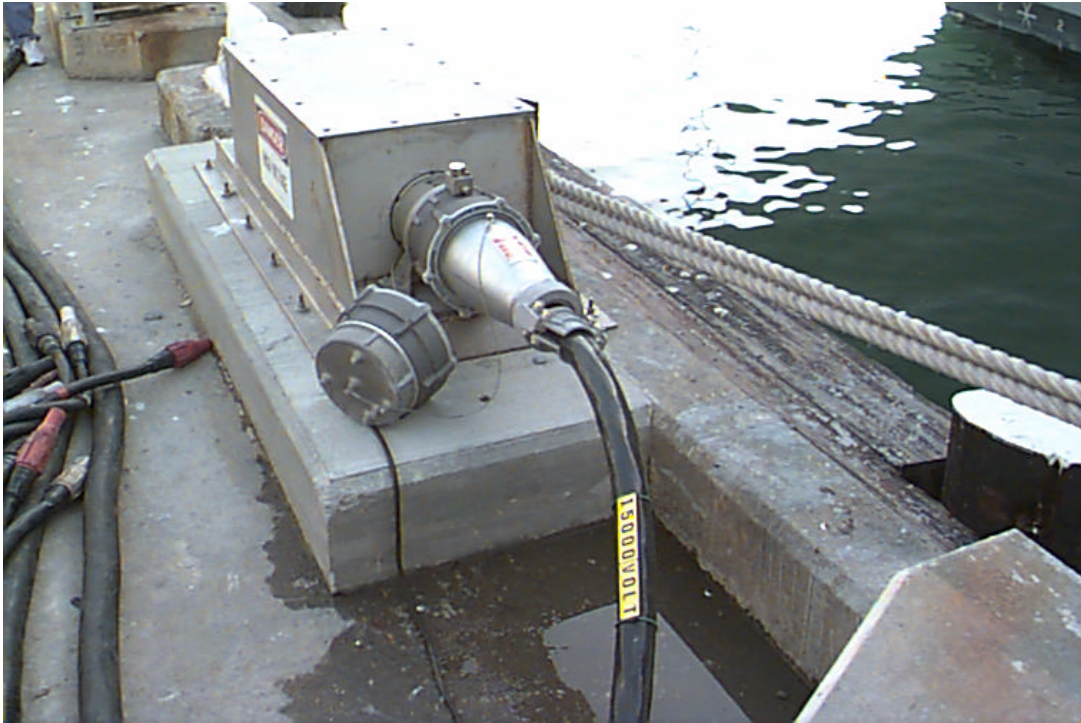
Picture A. Electrical connection outlet assembly with a 15-kV receptacle.
