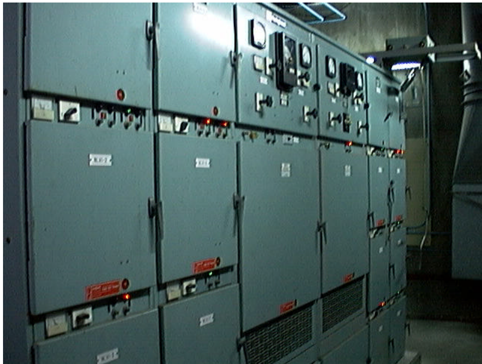
Picture B. Inside a pier vault housing a substation
