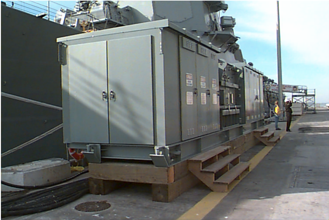
Picture C. A skid-mounted substation
