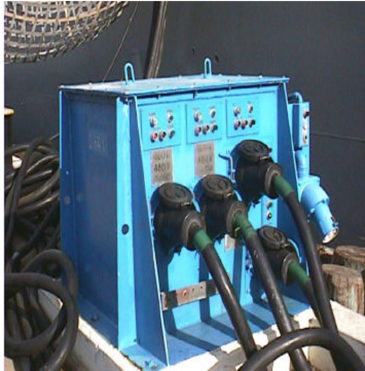
Picture G. A 480-volt pier electrical outlet assembly and cable connections.
