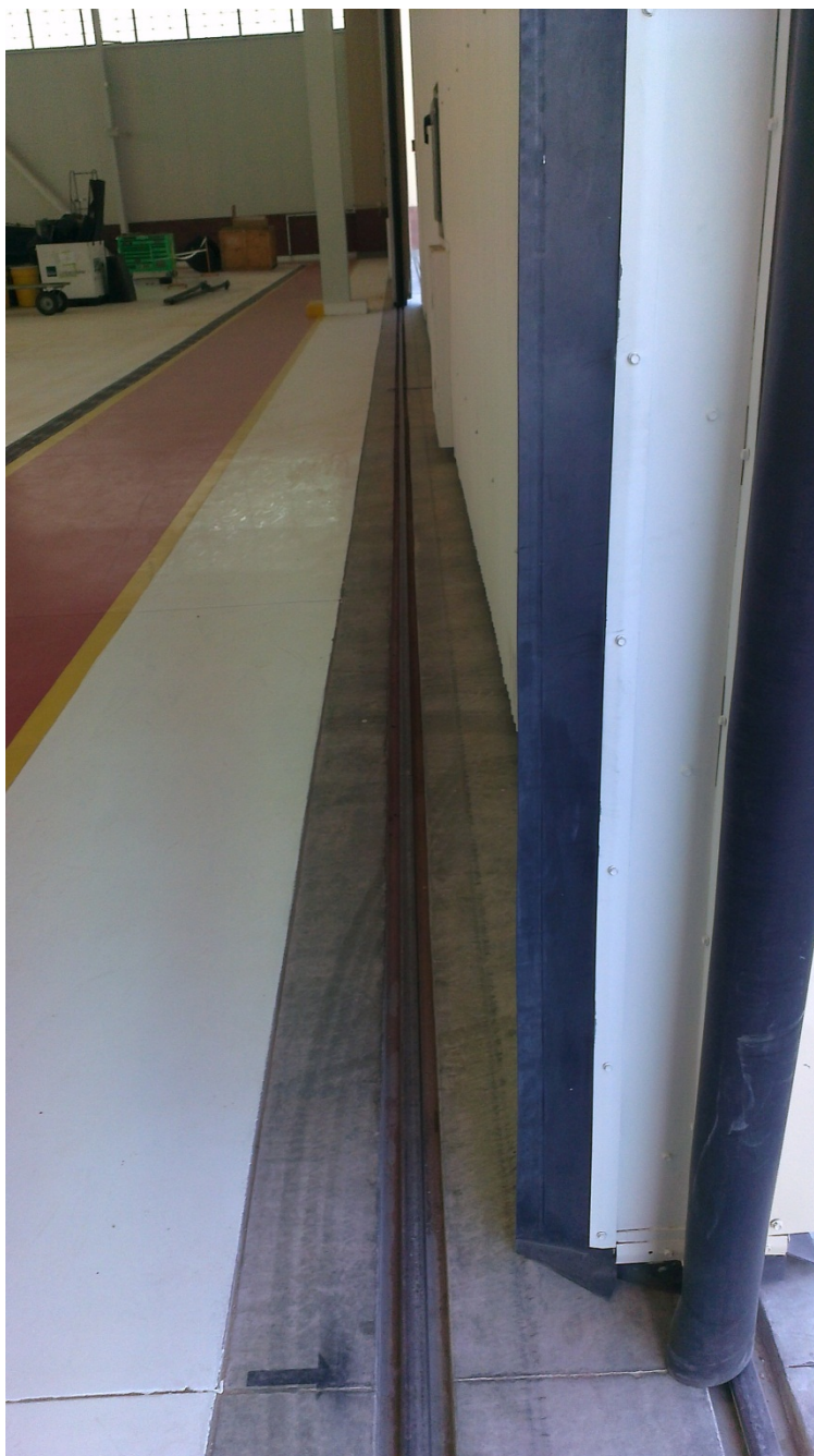
Figure E-12: Sliding Hangar Door Tracks
