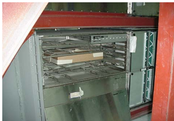
Figure G-6. Two 1,200-cfm M49 Assemblies Installed with HEPA Filters and Prefilters
