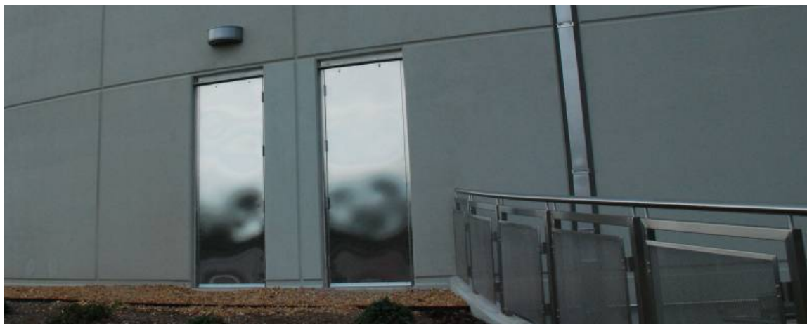
Figure 3-5 Emergency Exit Doors
