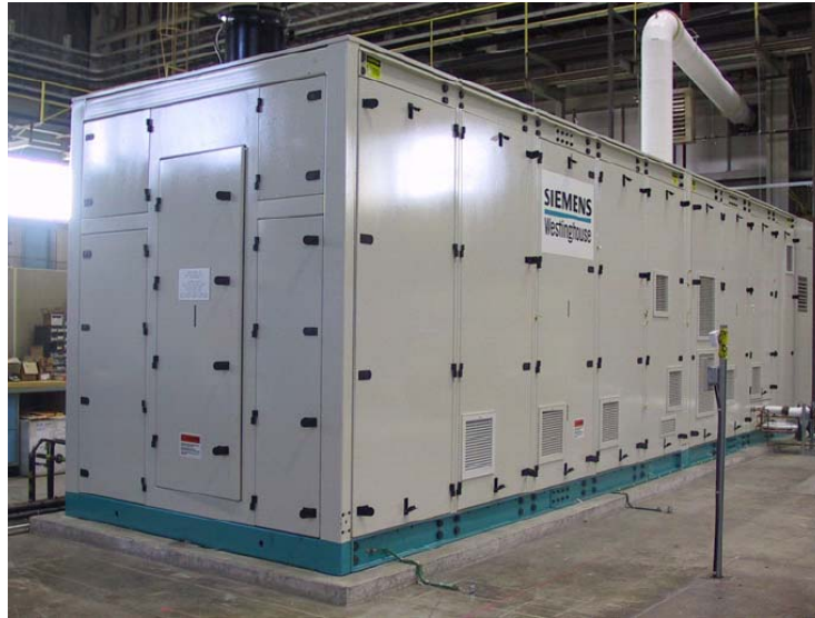
Figure 7-28 Siemens Westinghouse 250 kW Tubular SOFC Installation (31)
