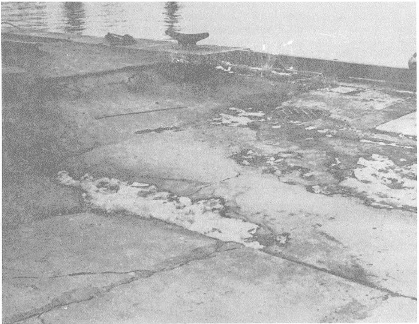
Figure 5-4. Cave-in, indicating settlement of mole.
