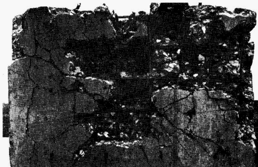
Fig. B-5 (b) Effect of 105-mm H.E. shell with concrete piercing fuze (rear view).
