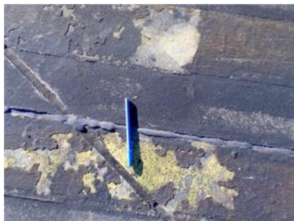
Example of Poor Joint Sealant
