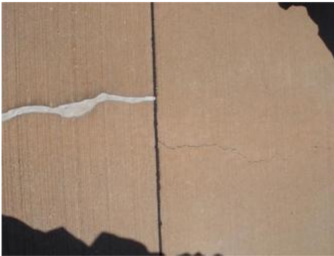
Example of Crack Repaired with Rout and Seal
