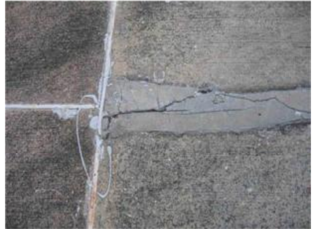
Example of “Poor” Concrete Repair
