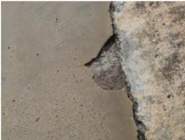
Example of Failed SRE Repair (where the material was too thin)
