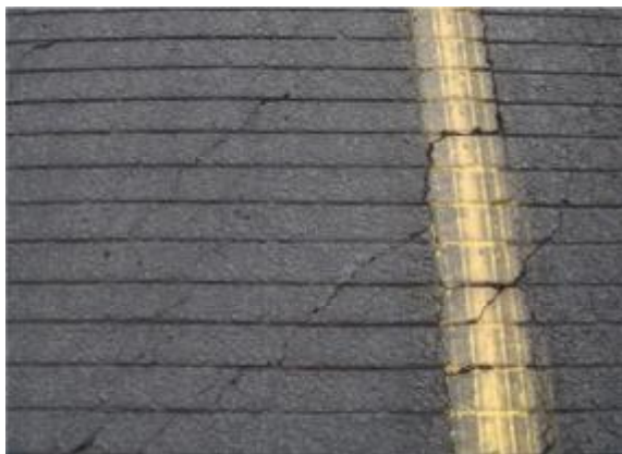
Example of High Severity Cracking
