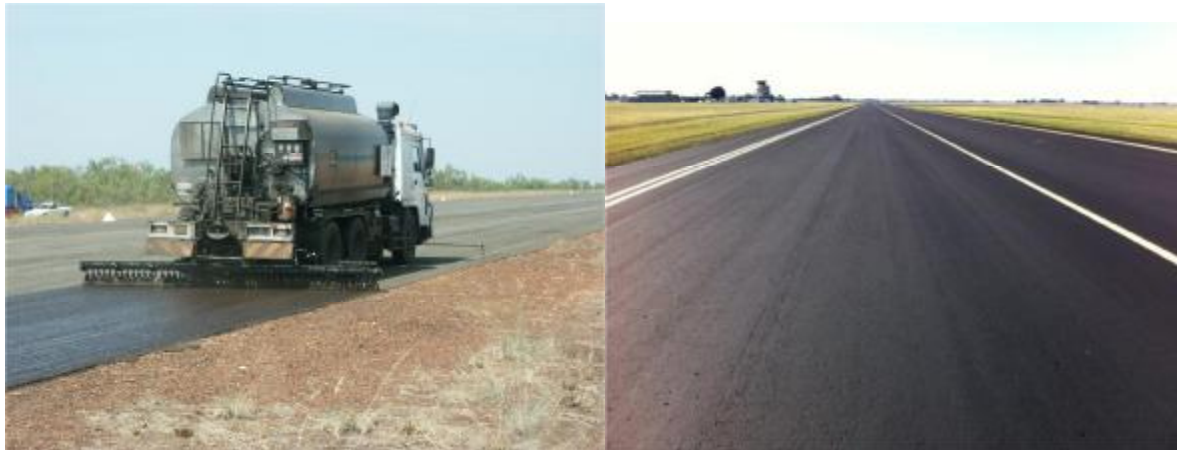
PME Application to Chip Seal Surface (Mount Bunday - August 2012) - Aged Asphalt - Pavement Treated with PME
