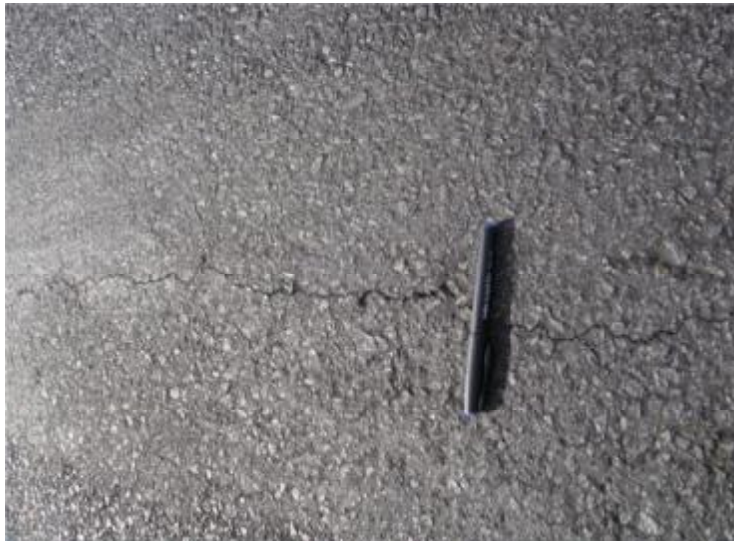
Example of Low Severity Cracking
