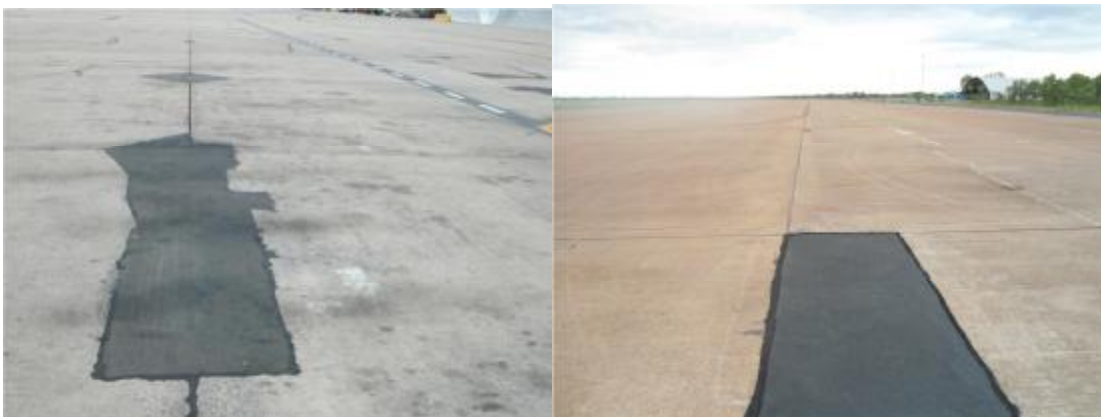
Examples of Hot Asphalt Joint and Corner Spall Repairs in Concrete Pavements
