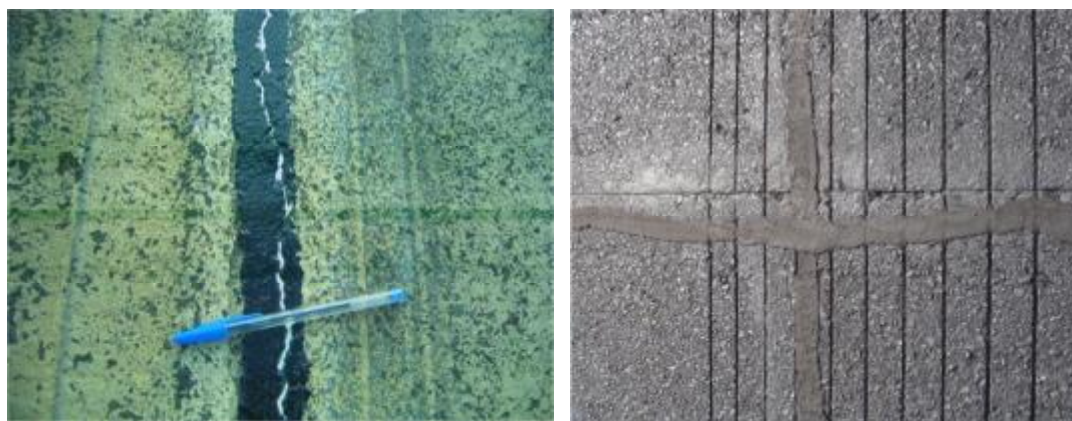
Examples of Poor Rubberised Bitumen Banding
