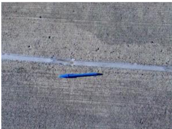
Example of Good Joint Sealant
